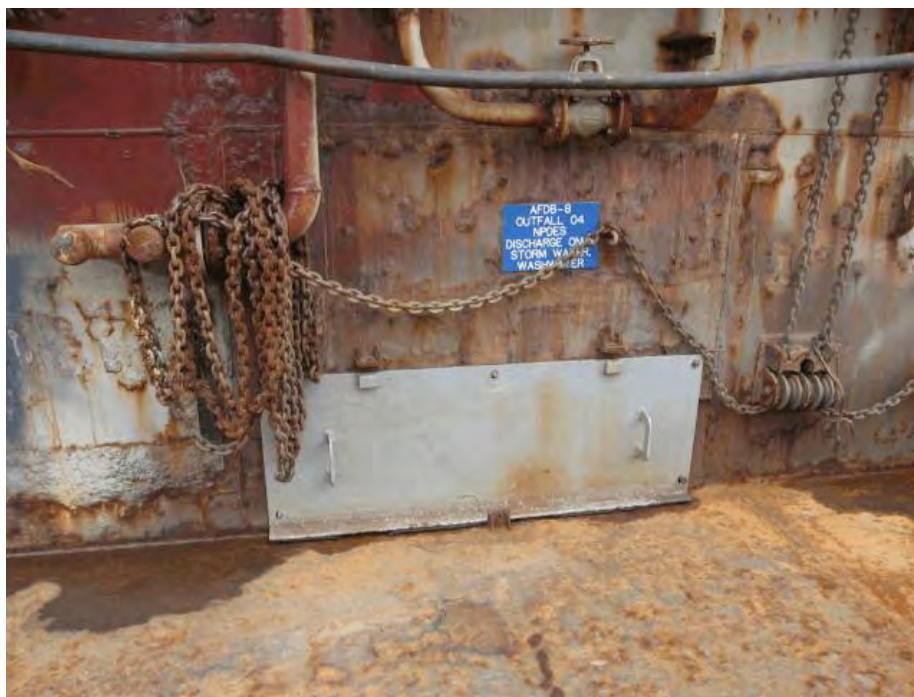
Photo 2 - View of Outfall No. 4 inlet on from inside drydock. Note metal plate used to prevent discharges during normal operations.
