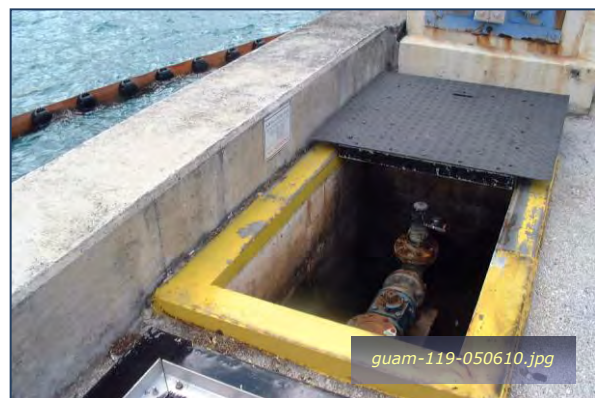
Photo #3-6: Victor Wharf - Bilge Pump Station Riser Taken By: Greg V. Arthur Date: 05/06/10
