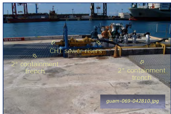
Photo #3-4: Echo Fueling Pier - CHT Sewer Riser Taken By: Greg V. Arthur Date: 04/28/10
