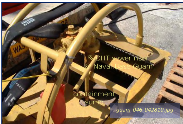
Photo #3-3: Sierra Wharf - CHT Sewer Riser Taken By: Greg V. Arthur Date: 04/28/10
