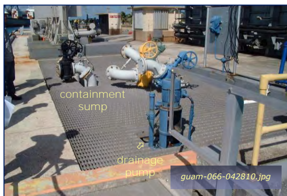
Photo #3-12: Delta Fueling Pier - Containment Sumps Taken By: Greg V. Arthur Date: 04/28/10
