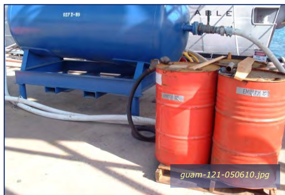
Photo #3-16: November Wharf – Condensate Capture Taken By: Greg V. Arthur Date: 05/06/10
