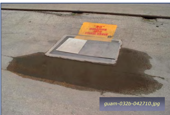
Photo #3-11: November Wharf - Covered Drain Taken By: Greg V. Arthur Date: 04/27/10
