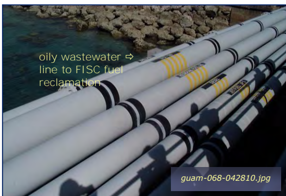
Photo #3-10: Fueling Piers - Bilge and Ballast Line Taken By: Greg V. Arthur Date: 04/28/10
