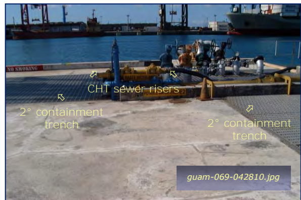
Photo #3-4: Echo Fueling Pier - CHT Sewer Riser Taken By: Greg V. Arthur Date: 04/28/10
