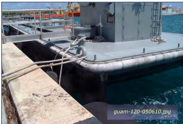
Photo #3-5: Victor Wharf - SWOB Bilge Barge Taken By: Greg V. Arthur Date: 05/06/10
