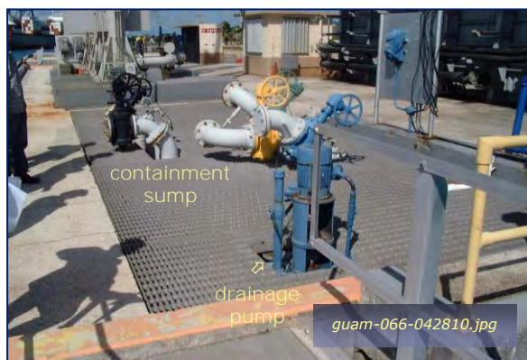
Photo #3-12: Delta Fueling Pier - Containment Sumps Taken By: Greg V. Arthur Date: 04/28/10
