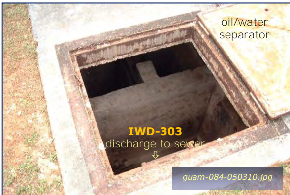
Photo #1-5: Hanger 3 - Oil Water Separator Taken By: Greg V. Arthur Date: 05/03/10
