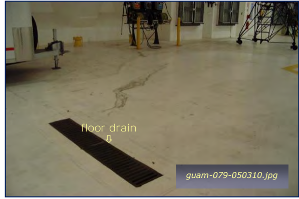
Photo #1-2: Hanger 2 - Floor Drain to O/W Sep Taken By: Greg V. Arthur Date: 05/03/10
