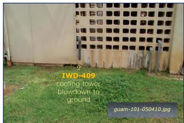
Photo #1-24: Bldg 25014 Chiller Plant - blowdown Taken By: Greg V. Arthur Date: 05/04/10
