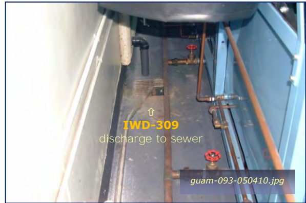
Photo #1-20: Bldg 17006 – NDT Discharge to Sewer Taken By: Greg V. Arthur Date: 05/04/10
