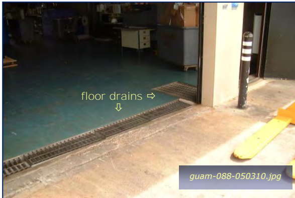
Photo #1-13: Bldg 19017 – Bay Door Drains Taken By: Greg V. Arthur Date: 05/03/10
