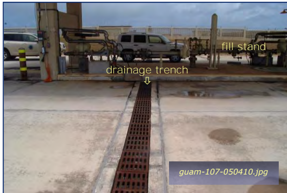
Photo #1-7: Satellite Fueling Station – Fill Stand Taken By: Greg V. Arthur Date: 05/04/10
