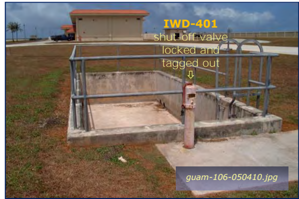
Photo #1-8: Satellite Fueling Station – Catchment Pit Taken By: Greg V. Arthur Date: 05/04/10
