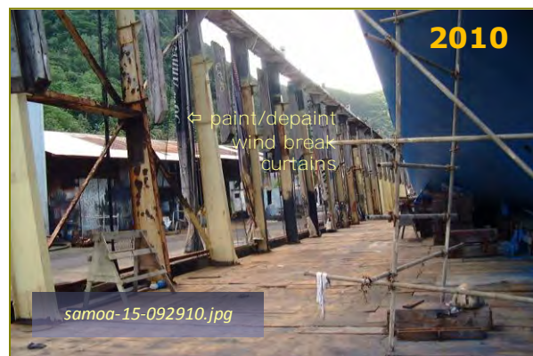
Photo #2: 3000-Ton Dry Dock – wind break curtains Taken By: Greg V. Arthur Date: 09/29/10
