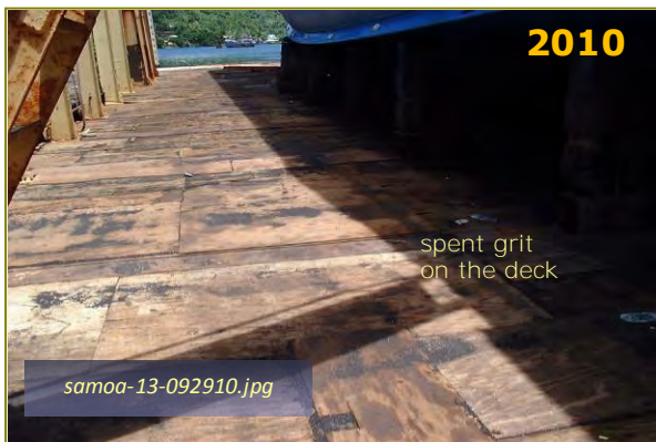
Photo #3: 3000-Ton Dry Dock Decking – Sept 2010 Taken By: Greg V. Arthur Date: 09/29/10
