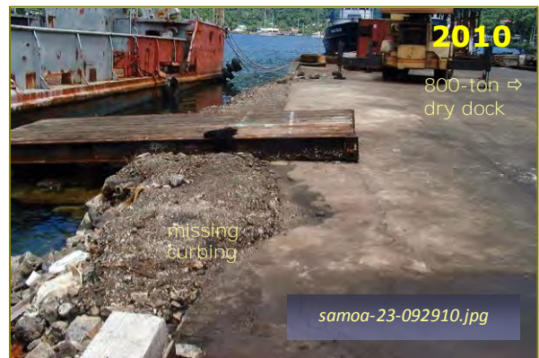
Photo #12: Catch Basin #1 - damaged waterfront Taken By: Greg V. Arthur Date: 09/29/10
