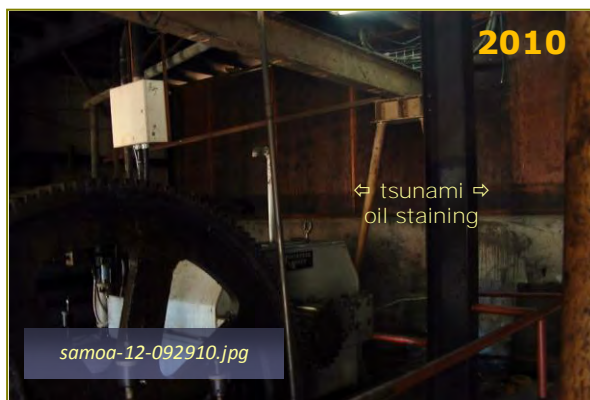
Photo #1: Engine Winch Room – 6' tsunami levels Taken By: Greg V. Arthur Date: 09/29/10
