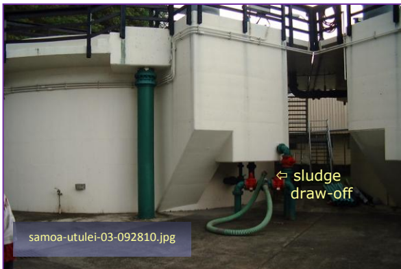
Photo #9: Utulei STP – Clarigester Sludge Draw-off Taken By: Greg V. Arthur Date: 09/28/10
