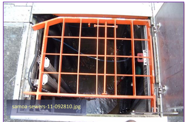
Photo #18: Fatumafuti Lift Station (To Utulei) Taken By: Greg V. Arthur Date: 09/28/10
