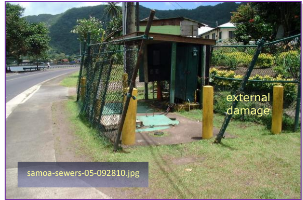
Photo #14: Satala Lift Station (Utulei service area) Taken By: Greg V. Arthur Date: 09/28/10
