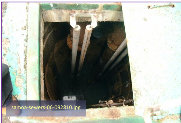
Photo #17: Korea House Lift Station (To Utulei) Taken By: Greg V. Arthur Date: 09/28/10
