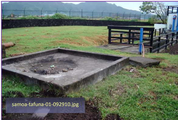
Photo #7: Tafuna STP – Septage Inlet Taken By: Greg V. Arthur Date: 09/29/10
