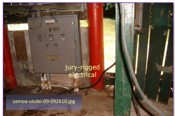
Photo #16: Malaloloa Main Lift Station (To Utulei) Taken By: Greg V. Arthur Date: 09/28/09
