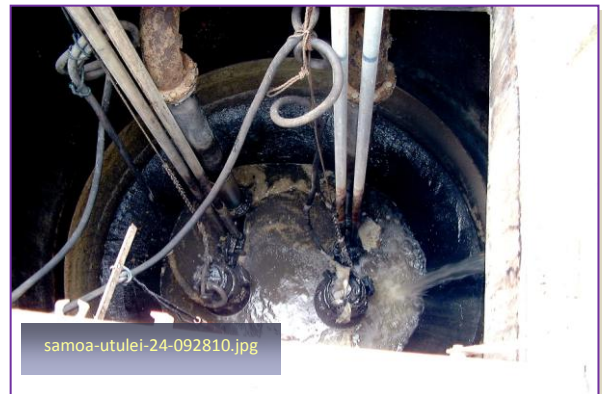
Photo #28: Airport Lift Station (Tafuna service area) Taken By: Greg V. Arthur Date: 09/28/10
