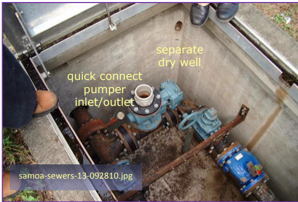
Photo #19: Fatumafuti Lift Station (To Utulei) Taken By: Greg V. Arthur Date: 09/28/10
