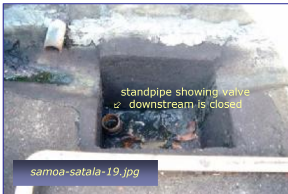
Photo #3: Drainage Sump within Fuel Tank Farm Taken By: Greg V. Arthur Date: 04/30/09
