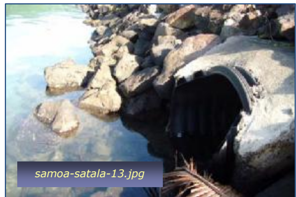
Photo #10: Culvert Outlet to the Harbor Taken By: Greg V. Arthur Date: 04/30/09
