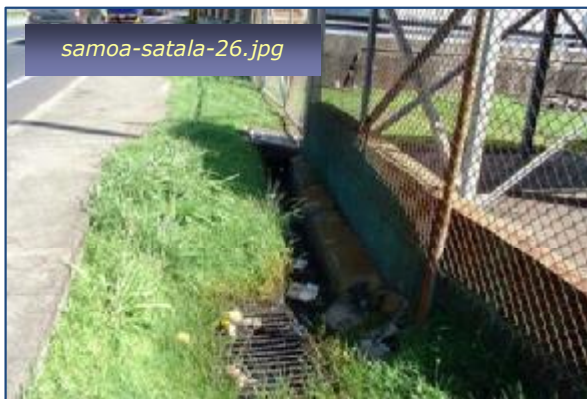
Photo #9: Storm Drainage Ditch - Culvert Inlet Taken By: Greg V. Arthur Date: 04/30/09
