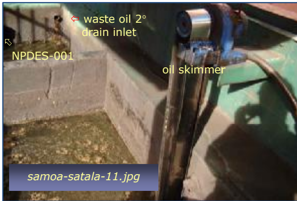
Photo #7: NPDES Sump #1 - Eastern Oil Water Sep Taken By: Greg V. Arthur Date: 04/30/09
