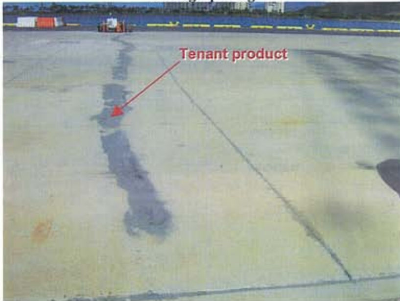
Photograph 21: At Piers 5 and 6 in Kalaeloa Barbers Point Harbor, tenant product had been spilled adjacent to a trench drain
