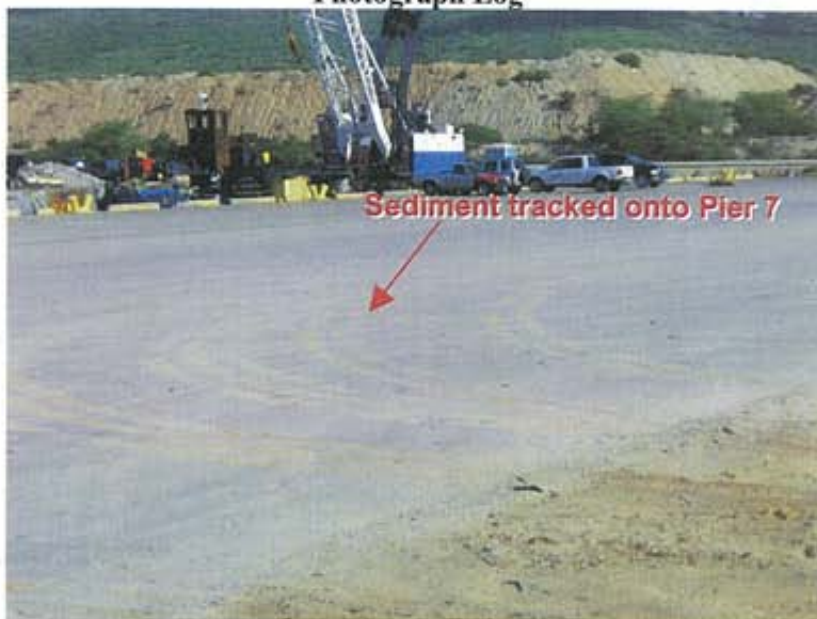
Photograph 7: Close-up view of area shown in Photograph 5 where sediment had been tracked onto the impervious pier surface
