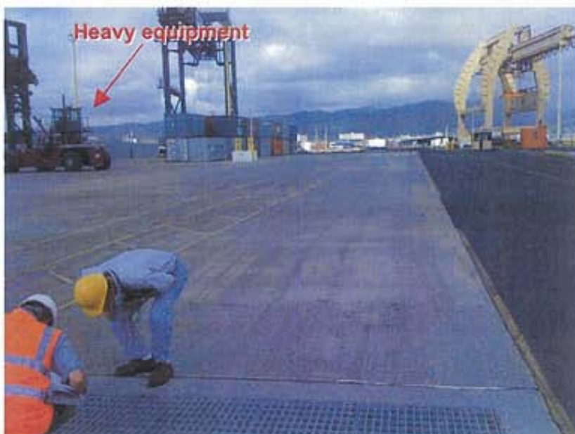
Photograph 18: View of trench drain where rubber material was observed
