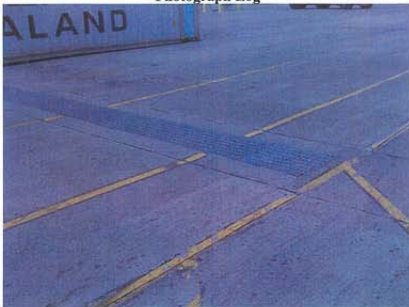
Photograph 17: Example of trench drain installed for storm drainage purposes
