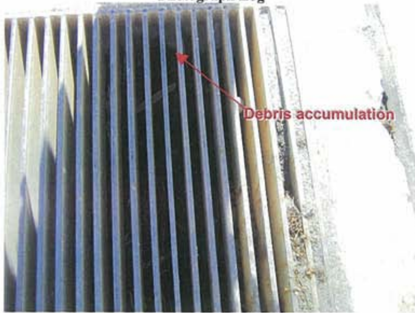
Photograph 23: At the location shown in Photographs 21 and 22, debris and/or tenant product had accumulated in the trench drain to nearly the top of the inlet grate
