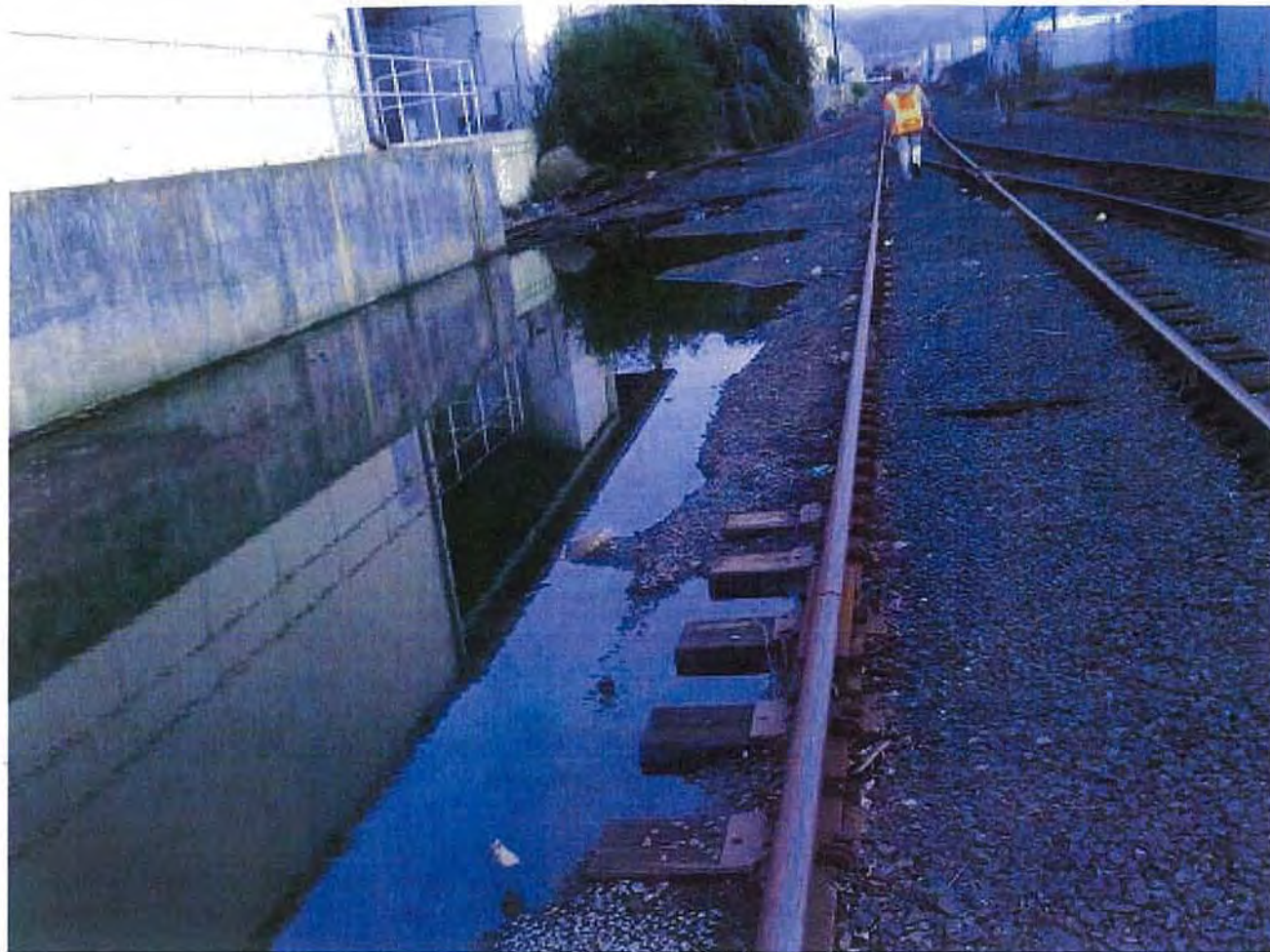
Storm water ponding rail spur 12-9-10
