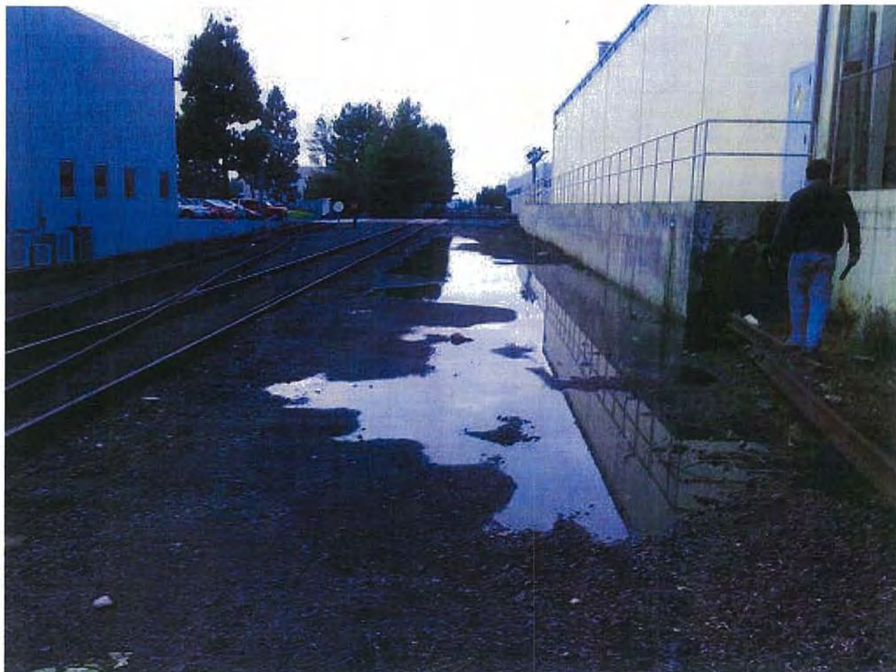
Storm water ponding due to drain cut at exit 12-9-10
