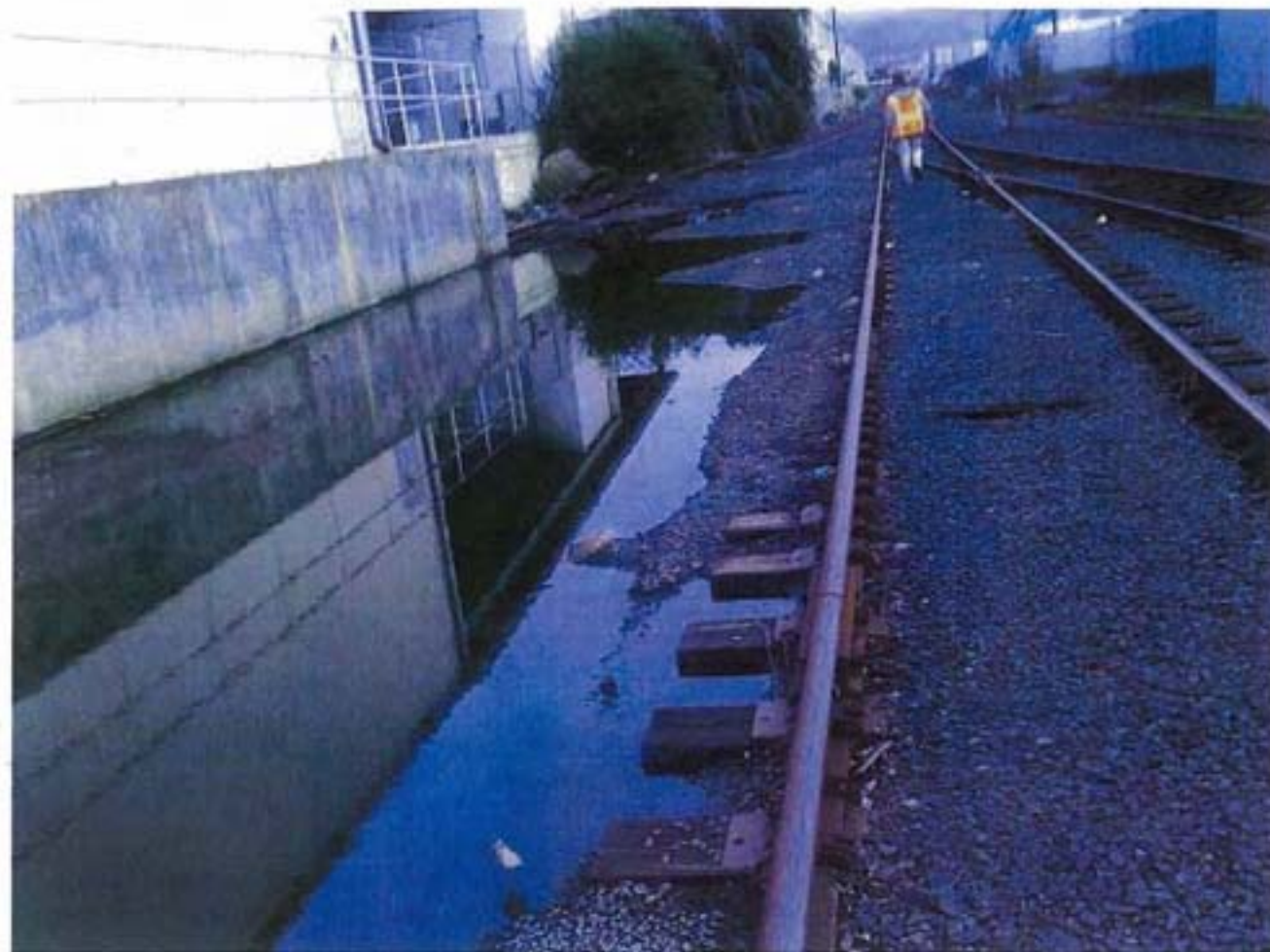
Storm water ponding rail spur 12-9-10
