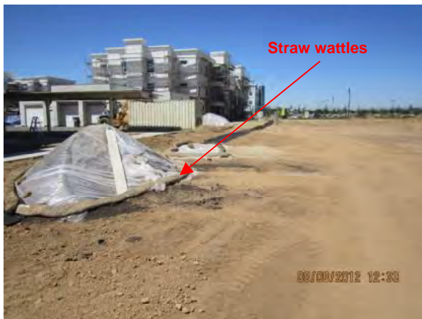
Photograph 3. View of stockpile along northern perimeter of the construction site. Note that the straw wattles placed around the stockpile were not entrenched into the ground.
