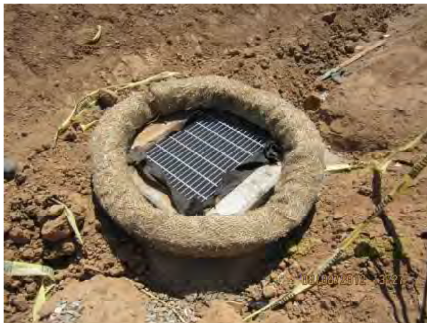
Photograph 9. Laguna Corporate Center Construction Project – Additional example of storm drain inlet in parking lot area surrounded by straw wattles which were not entrenched into the ground.
