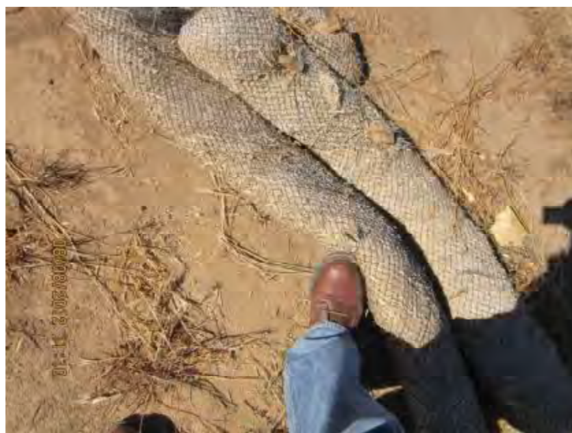
Photograph 4. Close-up view of straw wattles along the eastern edge of the site which were not entrenched into the ground.
