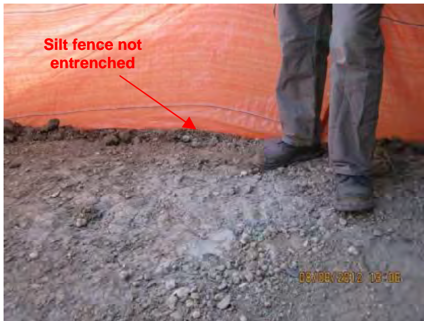
Photograph 2. Longleaf Drive Bridge Construction Project – Closer view of section of silt fence that was not entrenched into the ground noted in Photograph 1.
