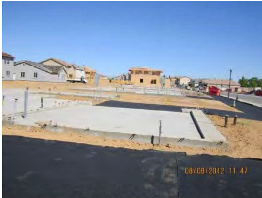
Photograph 1. View of lots with geotextile fabric applied around the perimeter of an active lot.
