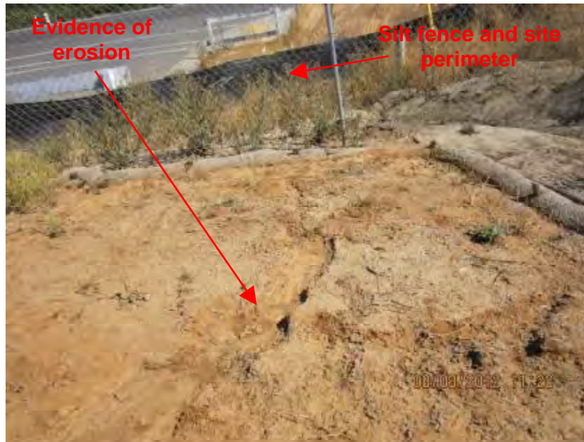
Photograph 5. View of straw wattle BMPs and silt fence BMP installed near the northeast corner of the site. Note evidence of erosion in foreground of the photograph.
