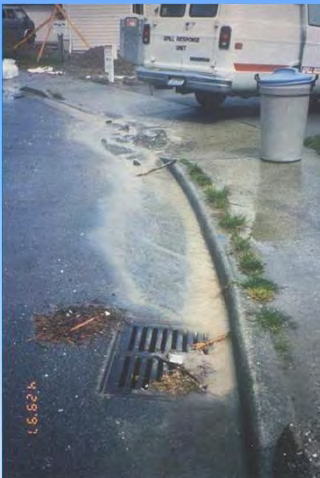
Illicit Discharge of Sediment Laden Water from Construction Site into Storm Drain Inlet
