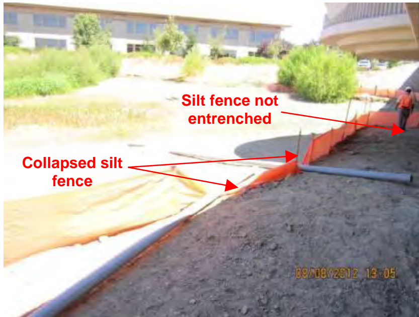
Photograph 1. Longleaf Drive Bridge Construction Project – View of area below the bridge where there was a section of collapsed silt fence and a section of silt fence that was not entrenched into the ground.
