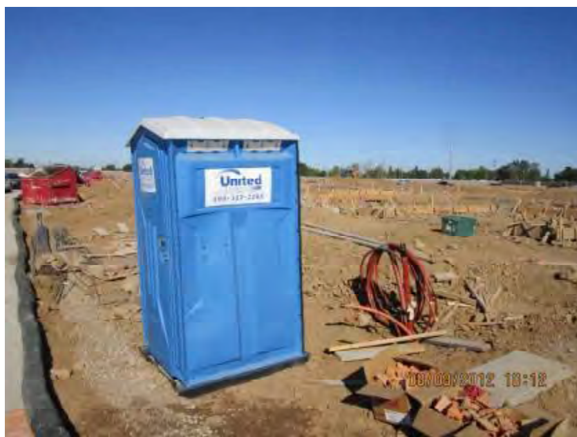
Photograph 4. View of an additional portable toilet at the site which was not staked into the ground or otherwise secured.
