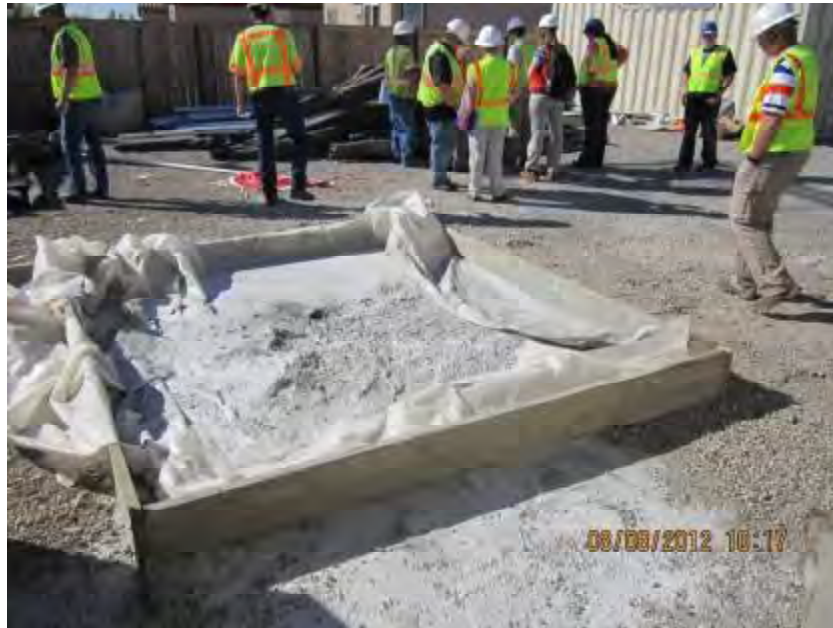
Photograph 5. View of concrete washout area at the site. Note concrete waste material located adjacent to the washout containment structure.
