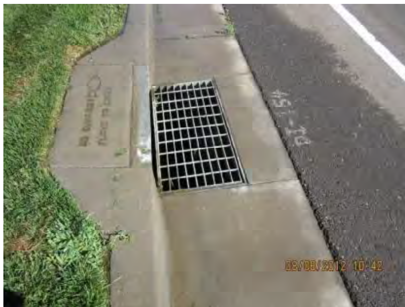
Photograph 6. Close-up view of storm drain inlet noted in Photograph 5. Note wetted area surrounding inlet.
