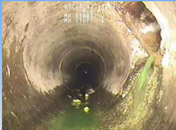
Illicit Connection identified by CCTV cameras
