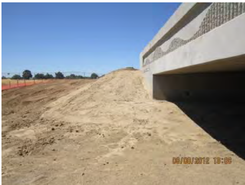
Photograph 4. Longleaf Drive Bridge Construction Project – View of south abutment on west side of the bridge. Note lack of erosion and sediment control BMPs.
