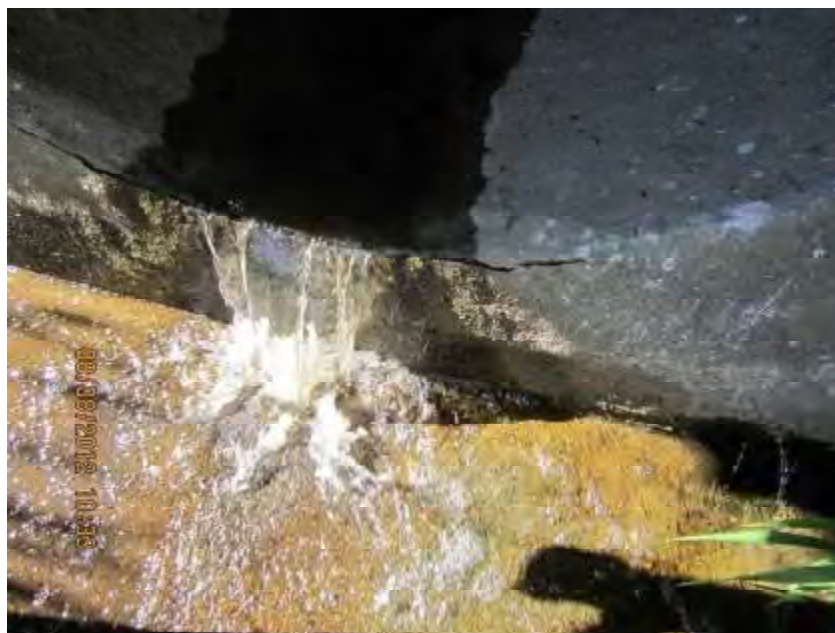
Photograph 4. Close-up view of dry weather flow from outfall.
