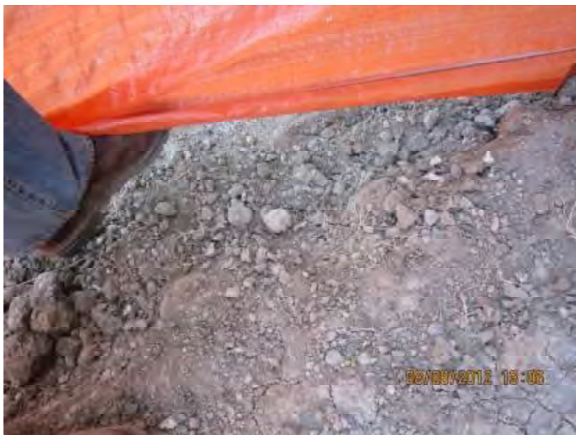
Photograph 3. Longleaf Drive Bridge Construction Project – Additional view of silt fence shown in Photographs 1 and 2 that was not entrenched into the ground.
