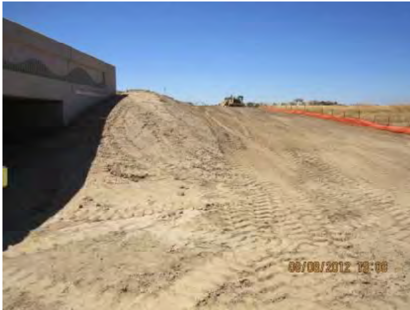
Photograph 5. Longleaf Drive Bridge Construction Project – View of north abutment on west side of the bridge. Note lack of erosion and sediment control BMPs.
