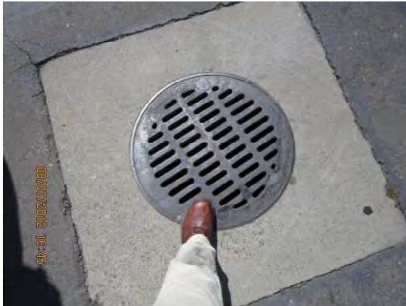
Photograph 11. View of storm drain inlet without BMPs for inlet protection.
