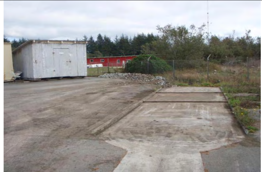
Photograph 6 – Area used for stockpiling washout material (Note: Sediment accumulation on impervious ground surface)
