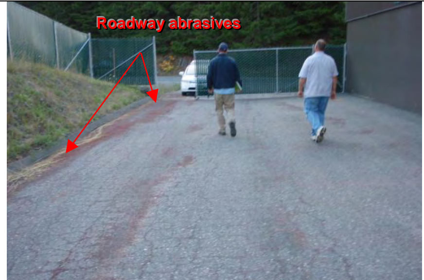
Photograph 6 – Roadway abrasives on impervious ground surface
