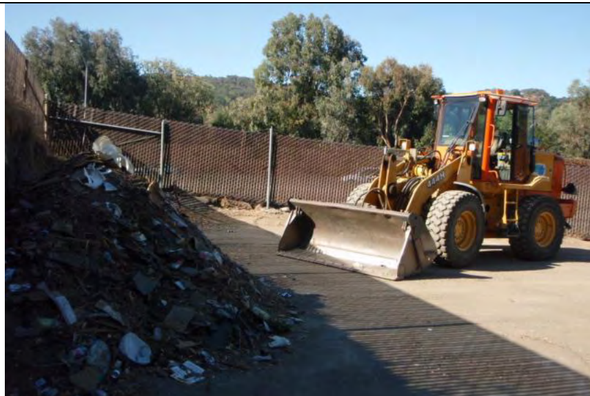
Photograph 2 – Waste from road sweeping and other road cleaning activities
