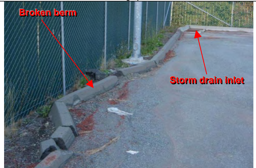
Photograph 4 – Broken berm along northern perimeter of facility (Note: Accumulation of roadway abrasives adjacent to berm)
