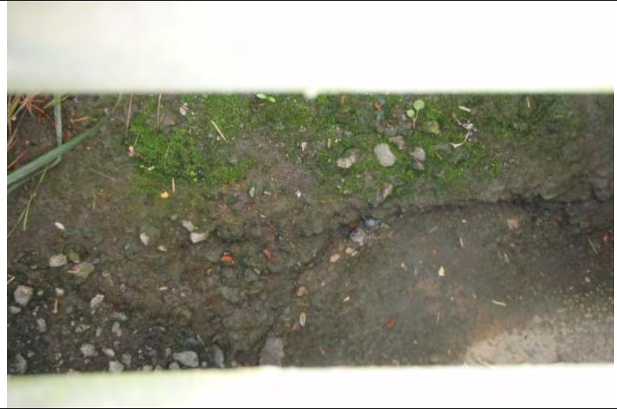
Photograph 2 – View into storm drain inlet pictured in Photograph 1 (Note: Sediment accumulation within inlet)
