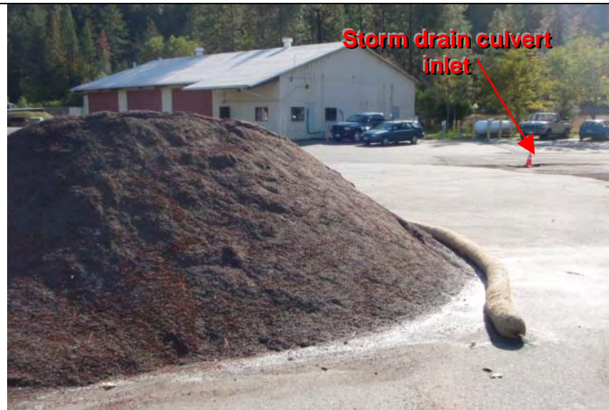
Photograph 6 – Inappropriate application of straw wattle BMP
