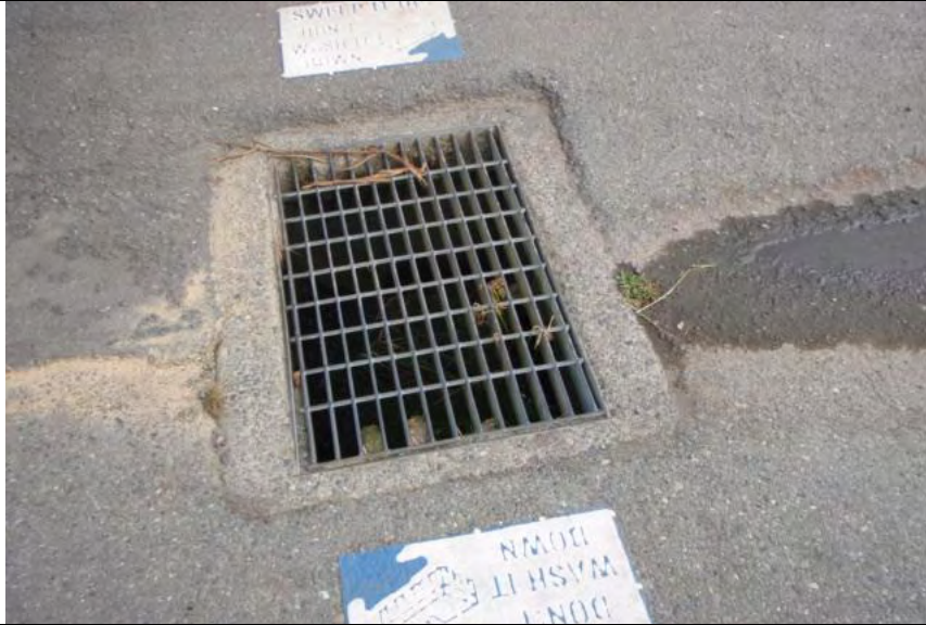
Photograph 1 – Storm drain inlet at facility
