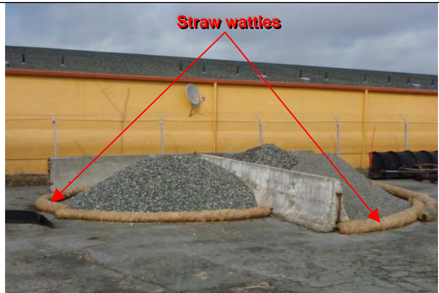
Photograph 10 – Inappropriate application of wattles on impervious surface
