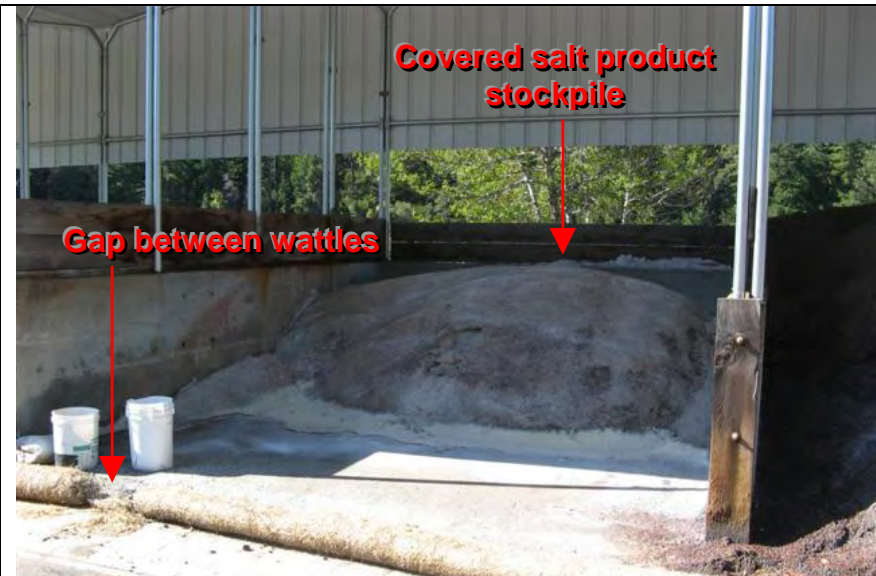
Photograph 9— Inappropriate application of wattles
