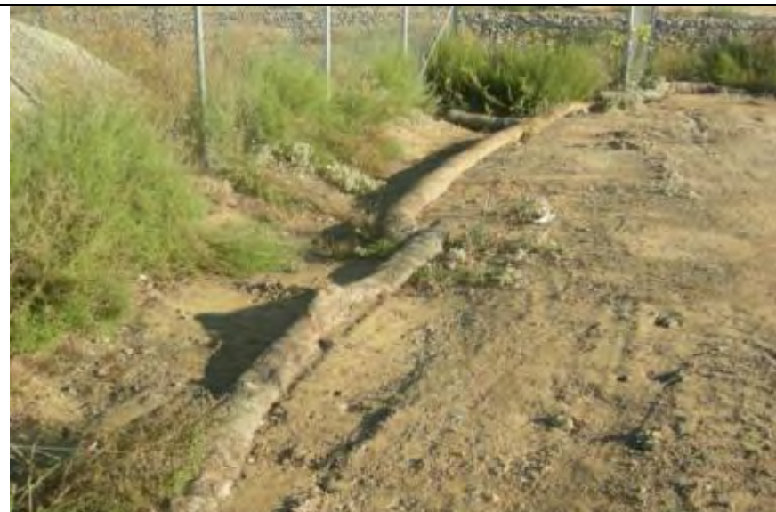
Photograph 2 – View of straw wattle BMPs, not adequately installed
