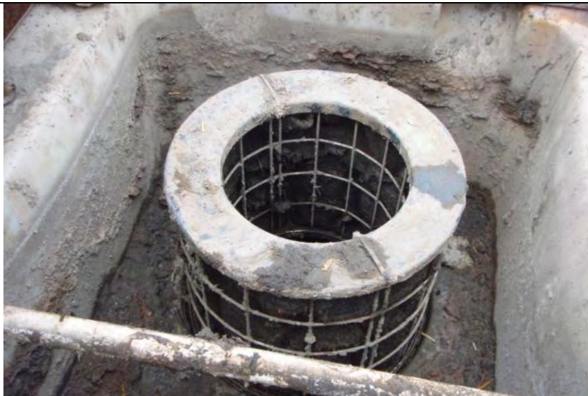
Photograph 9— Closer view of filter shown in Photograph 8. (Note: Pollutant accumulation within filter and inlet)
