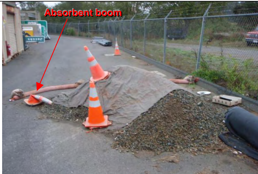
Photograph 10 – Partially covered and contained stockpile along eastern edge of facility
