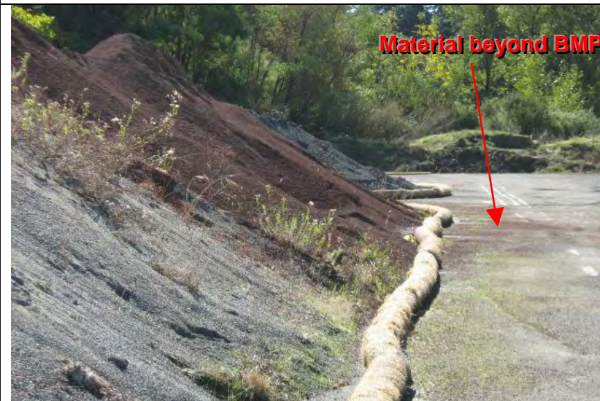
Photograph 8 – Inappropriate application of wattles on impervious surface
