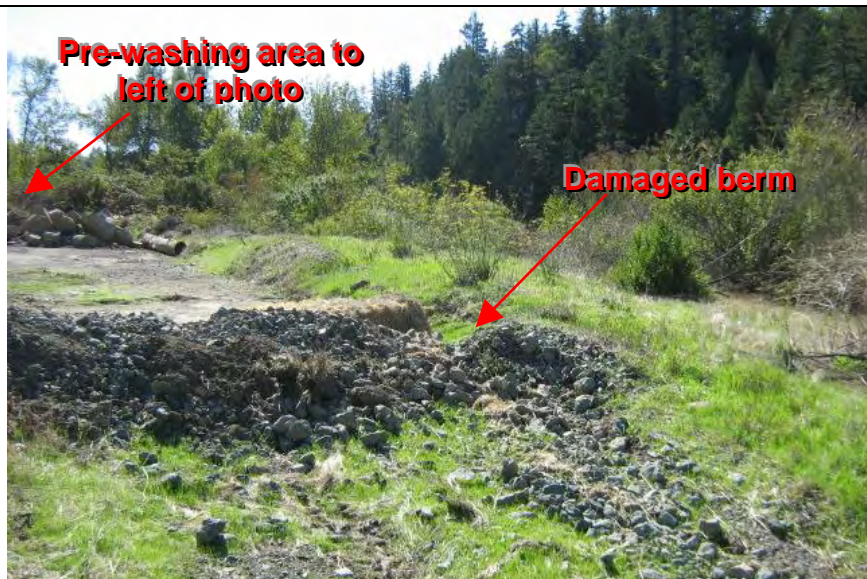
Photograph 7— Damaged berm shown in Photograph 6
