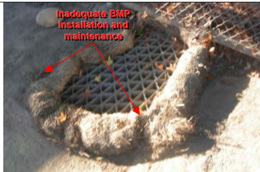
Photograph 4 – Storm drain inlet on the east side of the Marysville Maintenance Station office building
