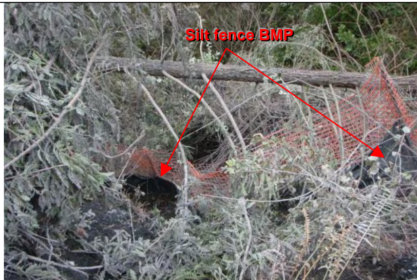
Photograph 6 – Example of silt fence BMP partially covered by collapsed vegetation
