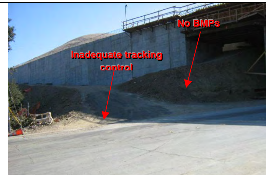
Photograph 8 – View of fill slope along access road without BMPs and vehicle tracking control pad
