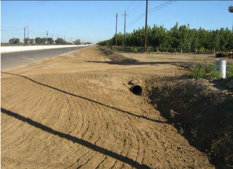
Photograph 1 – Drainage swale adjacent to roadway without adequate BMPs implemented (Drill seeding only)
