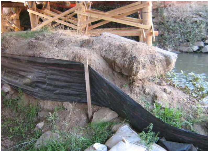
Photograph 11 – Silt Fence BMPs not properly installed (e.g., not entrenched) or maintained (e.g., collapsed) adjacent to Auburn Ravine
