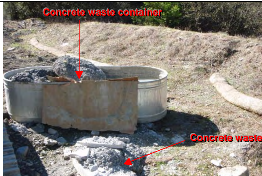
Photograph 10— Concrete waste and container in staging area (Note: Straw wattle BMP not staked or entrenched into ground)
