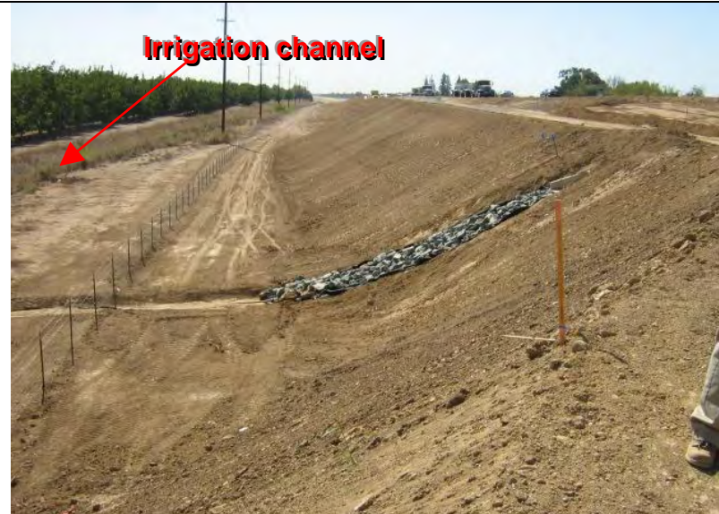
Photograph 26 – Large expanse of disturbed slope area with only rock and no perimeter BMPs.
