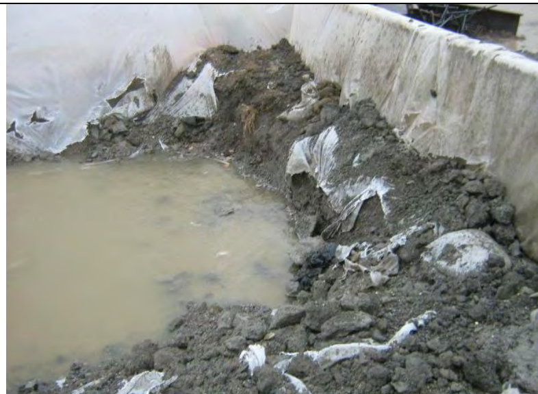
Photograph 2 – Close-up view of unmaintained (e.g., torn and deteriorated) concrete washout plastic liner
