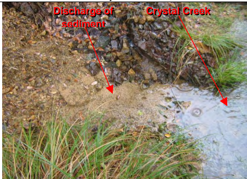
Photograph 7—Visible evidence of the discharge of sediment from the upgradient disturbed slope areas to Crystal Creek
