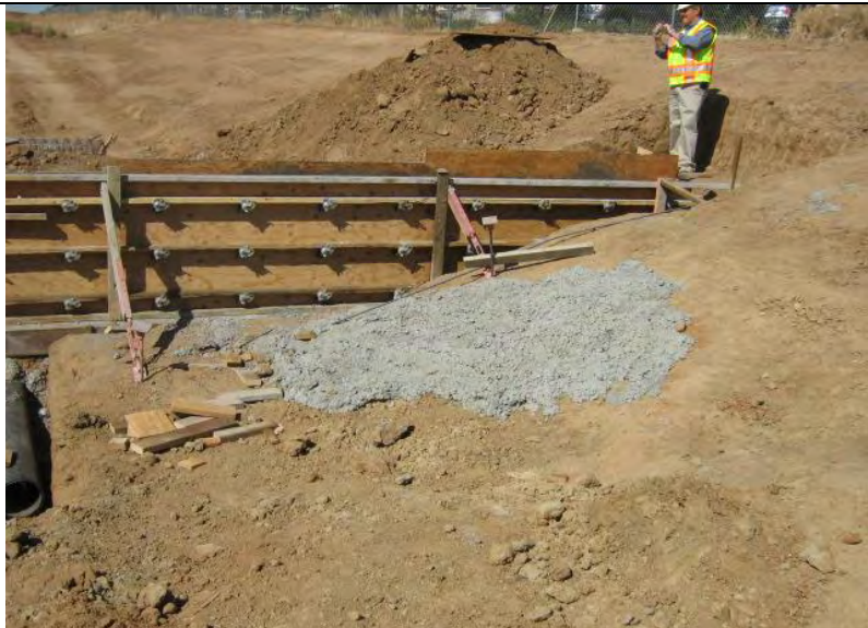
Photograph 1 – Improper concrete waste disposal practices
