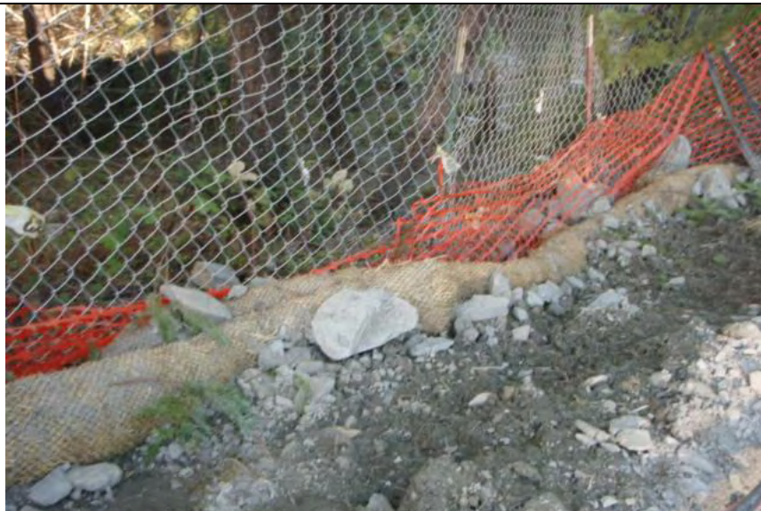
Photograph 5— Example of sediment and debris accumulation against straw wattle BMP
