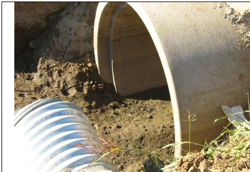
Photograph 9 – Visible sediment accumulation in the irrigation channel and associated culvert pipe
