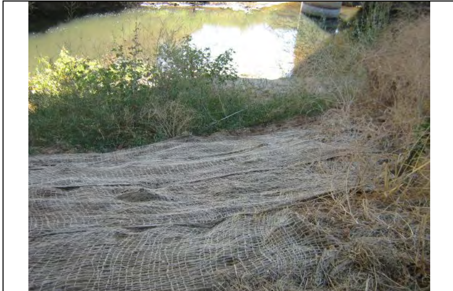
Photograph 1 – Erosion control blanket not properly installed (e.g., improper overlap – not shingled downgradient) adj. to Bear River at top.
