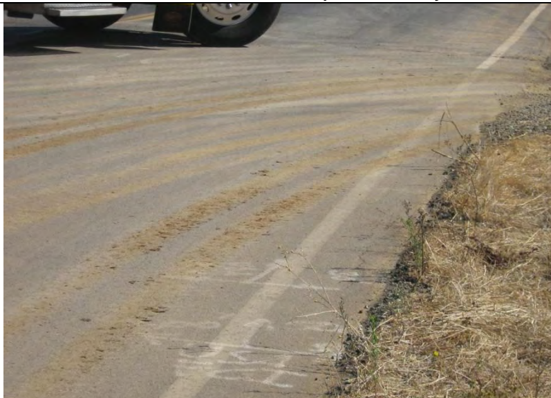
Photograph 15 – Sediment transport from areas of disturbance onto Feather River Boulevard, a public roadway.
