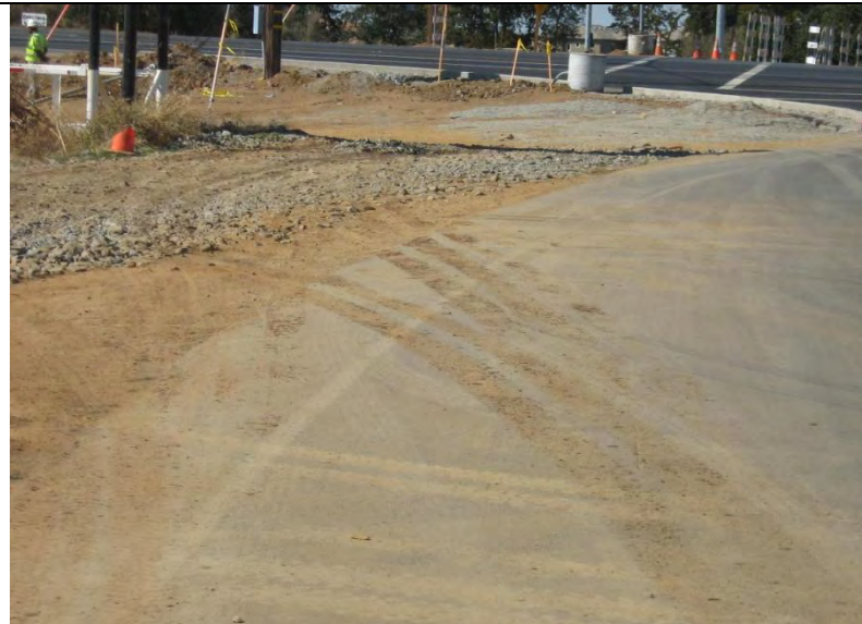
Photograph 14 – Sediment transport from areas of disturbance onto Feather River Boulevard, a public roadway.
