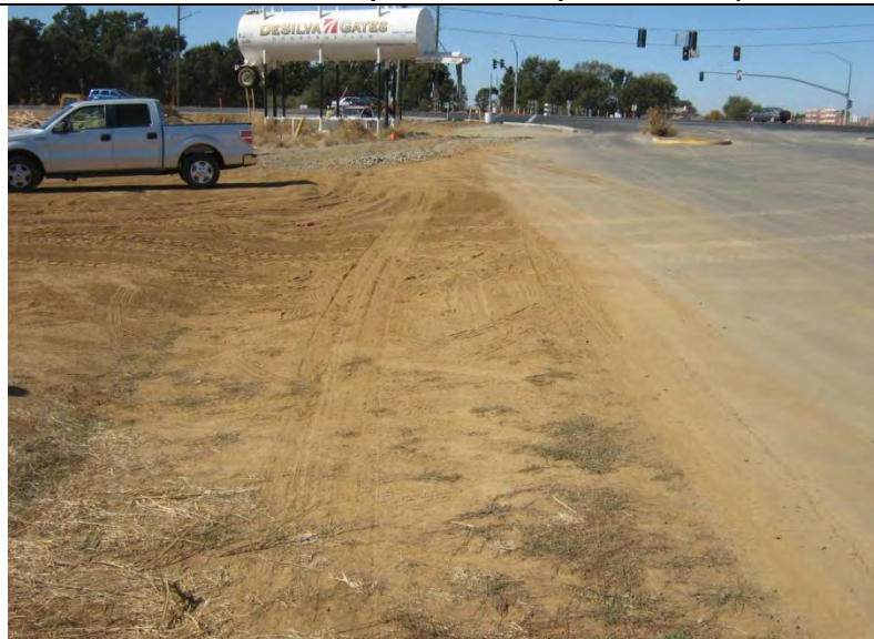
Photograph 12 – Tracking control BMPs not implemented for disturbed area of contractor parking. Observed sediment transport to roadway
