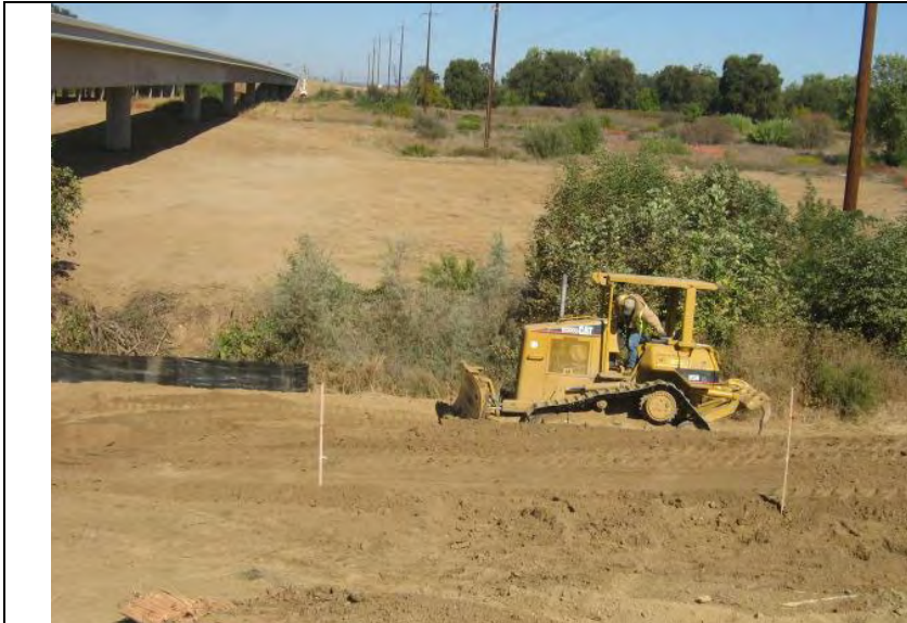
Photograph 25 – SF not adequately implemented for all land disturbing activities to prevent the discharge of sediment to Yankee Slough
