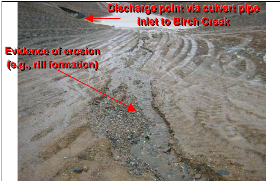
Photograph 5— Close-up of area in Photograph 4 depicting erosion (e.g., rill formation) and inadequate BMPs located adjacent to discharge point
