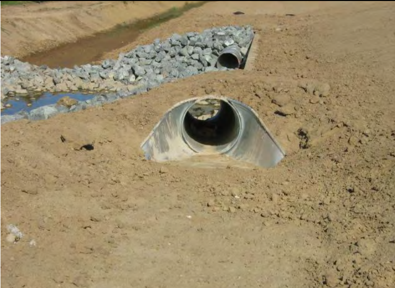
Photograph 15 – Inlet protection BMPs were not implemented for a culvert inlet draining to the irrigation channel.
