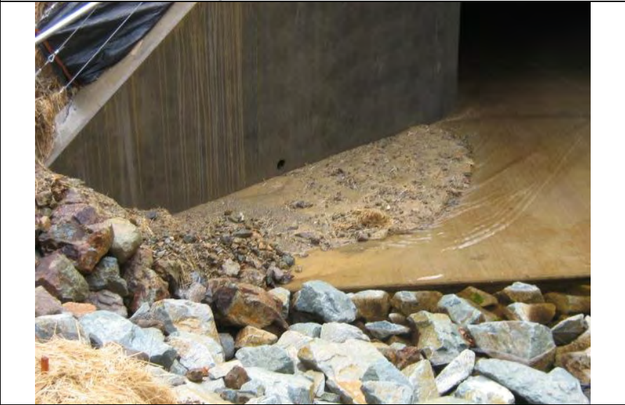
Photograph 12 – Close-up view of Photograph 11 depicting the discharge of sediment and sediment accumulation in Yankee Gulch
