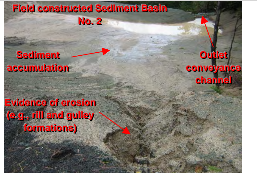
Photograph 10 – Evidence of the discharge of sediment to the basin and sediment accumulation in the basin which drains to unnamed tributary
