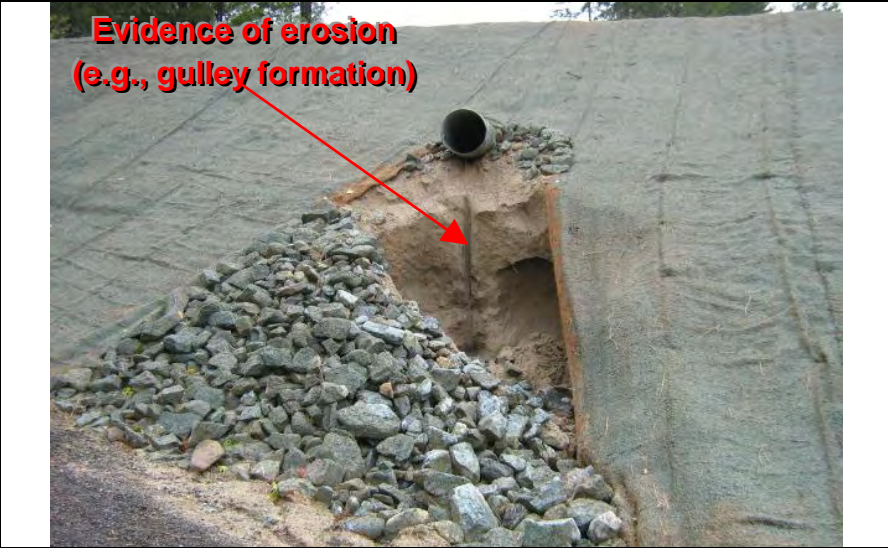
Photographs 16 – Adequate BMPs were not implemented below field constructed sediment basin No. 1 culvert outlet pipe.
