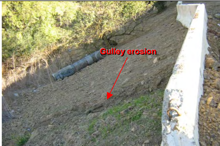
Photograph 3 – Slope erosion below undercut K-rail shown in Photograph 2
