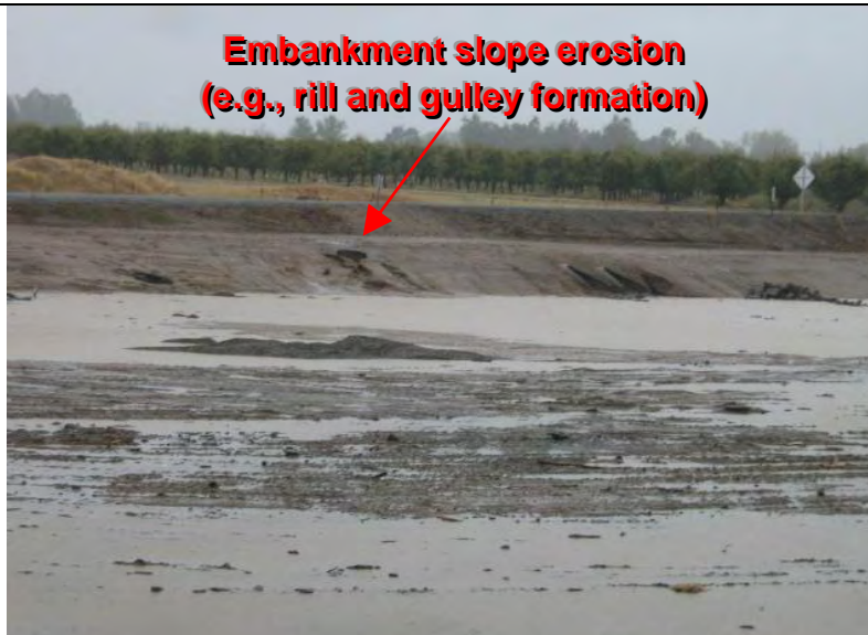
Photograph 2 – Erosion of unstabilized sediment basin and associated embankment slopes
