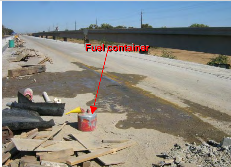
Photograph 18 – Inadequate materials handling and storage
