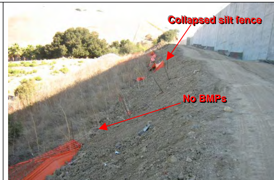
Photograph 6 – Fill slope along access road without BMPs
