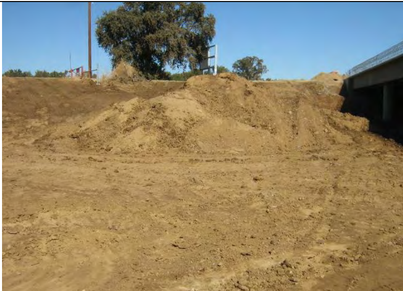
Photograph 5 – Soil stockpile with no perimeter controls or temporary stabilization located just upgradient of Bear River crossing.
