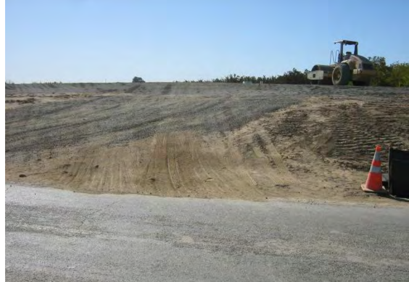
Photograph 20 – Adequate tracking control BMPs had not been implemented at the Wilson Road intersection.
