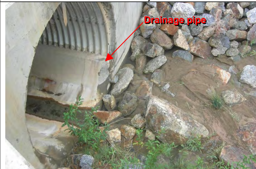
Photograph 7 – Sediment accumulation at down-gradient drainage pipe inlet
