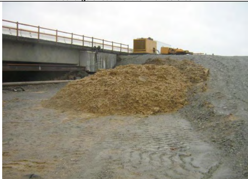
Photograph 11— Soil stockpile without BMPs
