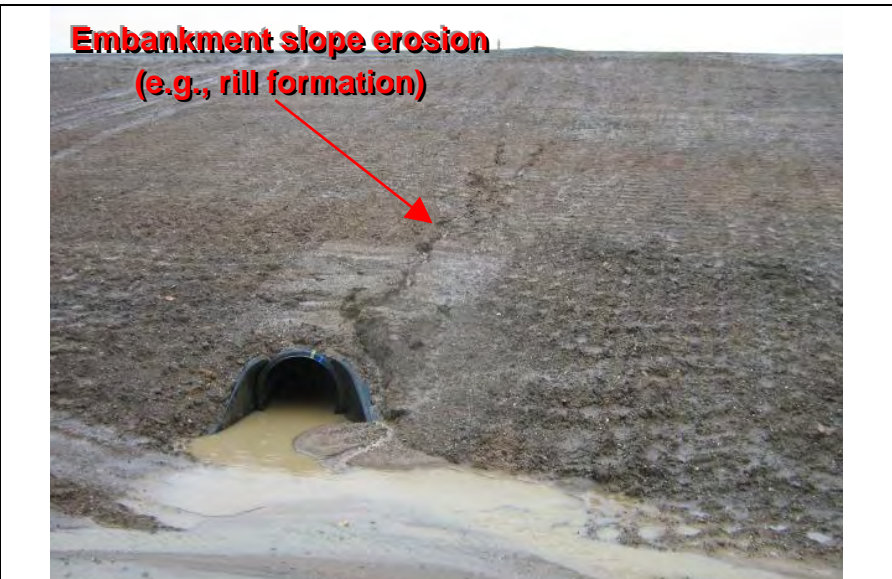
Photograph 6 – Embankment slope erosion (e.g., rill formation)
