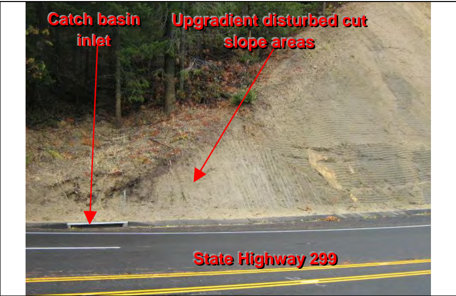
Photographs 22 – BMPs were not implemented to prevent the discharge of sediment from upgradient disturbed cut slope areas to catch basin inlets.
