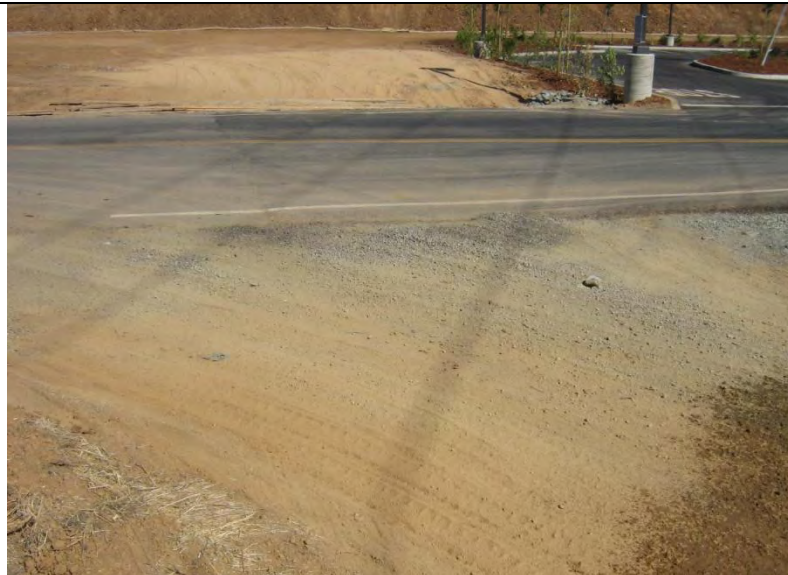
Photograph 10 – Tracking control BMPs not adequately maintained (e.g., sediment in rock pad and rock sparse in areas)
