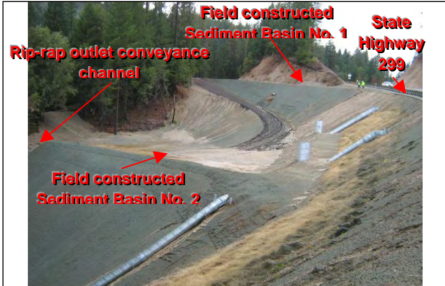
Photograph 9—Vantage point photograph depicting location of field constructed sediment basins No. 1 and No. 2 and their outlet.
