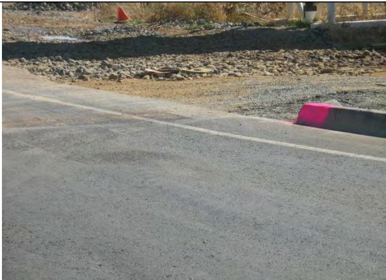
Photograph 11 – Tracking control BMPs not adequately maintained (e.g., sediment in rock pad and rock sparse in areas)
