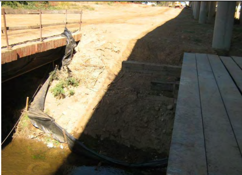
Photograph 21 – Silt Fence BMP not properly maintained (e.g., collapsed) adjacent to Yankee Slough. Note area of disturbance up-gradient.
