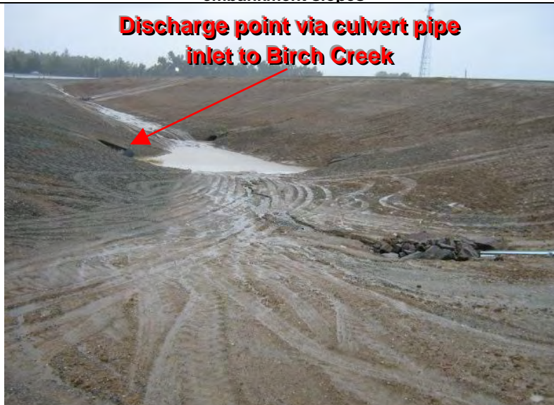
Photograph 4 – Adequate BMPs had not been implemented to prevent the discharge of sediment to the culvert inlet/drainage pipe leading to Birch Cr.
