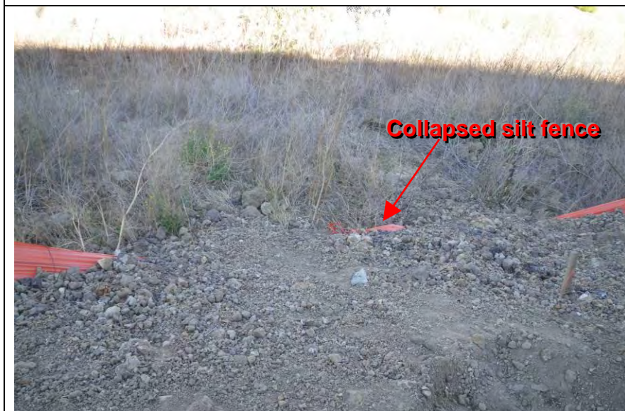
Photograph 7— Collapsed silt fence due to slide
