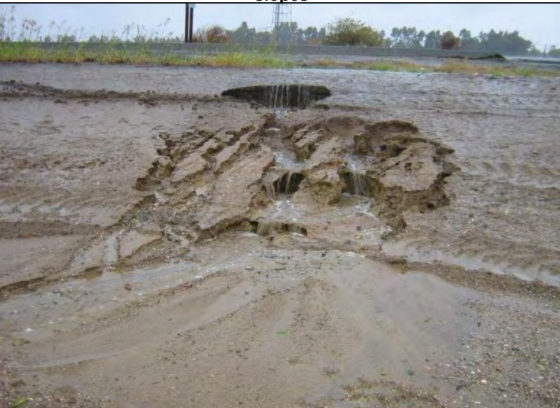
Photograph 3 – Sediment basin embankment slope erosion (e.g., gully formation) and failure
