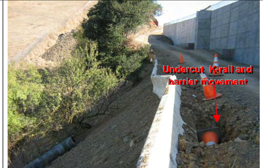
Photograph 2 – Failed fill slope along access road
