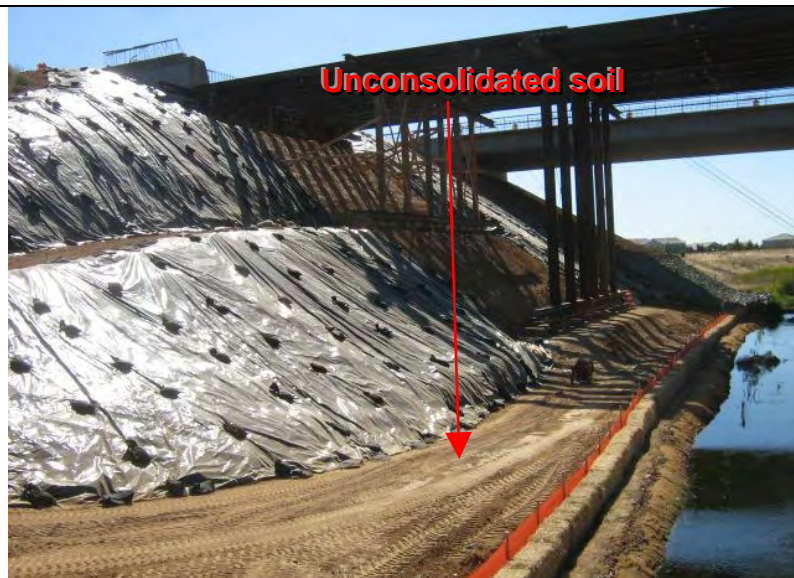
Photograph 4 – No BMPs to control concentrated flow off of the plastic and across the unconsolidated material at the toe of the slope
