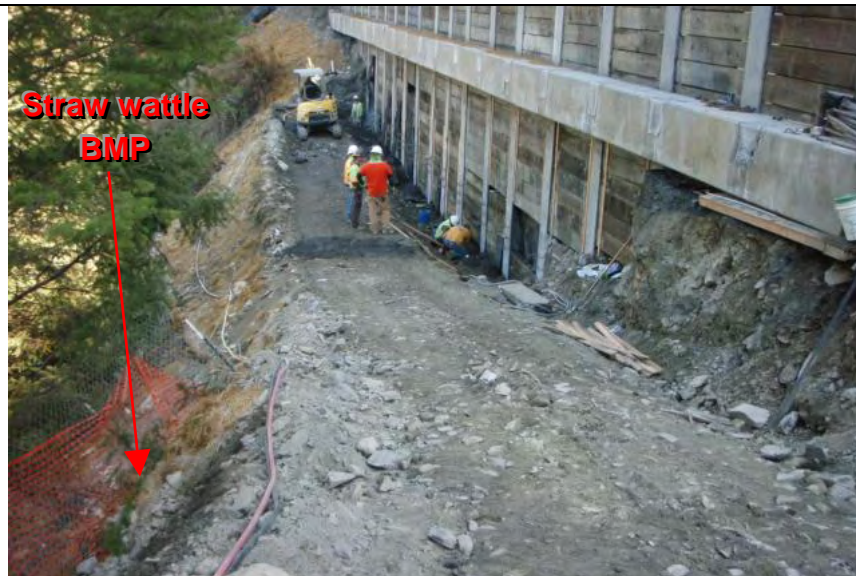
Photograph 2 – Example of straw wattle BMP implemented down-gradient of disturbance and retaining wall construction
