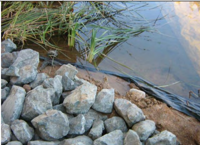
Photograph 7 – Badly deteriorated silt fence BMP located in/adjacent to North Ingram Slough
