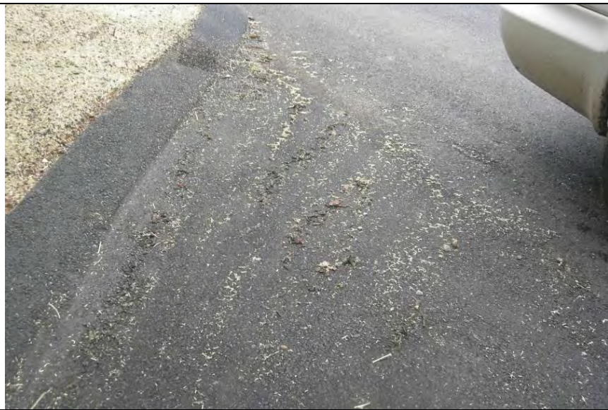
Photograph 3 – Sediment and debris from Photograph 2
