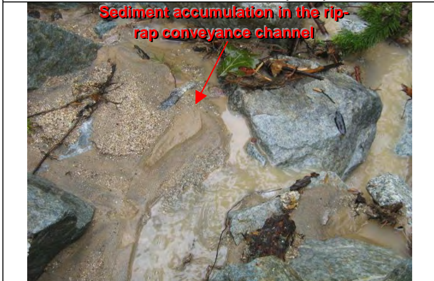
Photograph 7—Visible evidence of sediment accumulation in the rip-rap outlet conveyance channel which drains to the unnamed tributary
