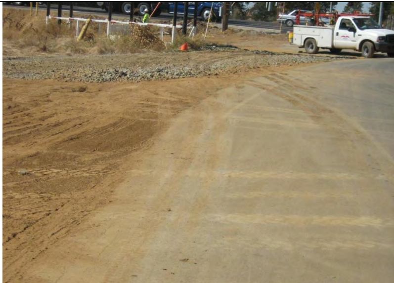
Photograph 13 – Sediment transport from areas of disturbance onto Feather River Boulevard, a public roadway.
