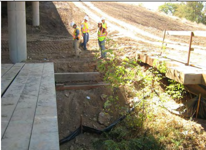
Photograph 23 – Silt Fence collapsed in areas and not properly maintained. Note large unstabilized slope area upgradient.
