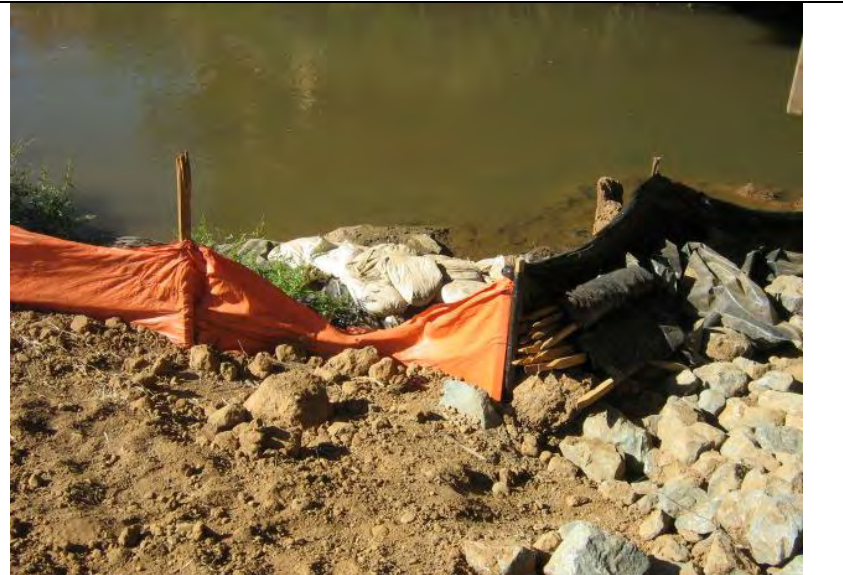
Photograph 14 – Silt Fence BMP not adequately maintained (e.g., down in areas) adjacent to Auburn Ravine
