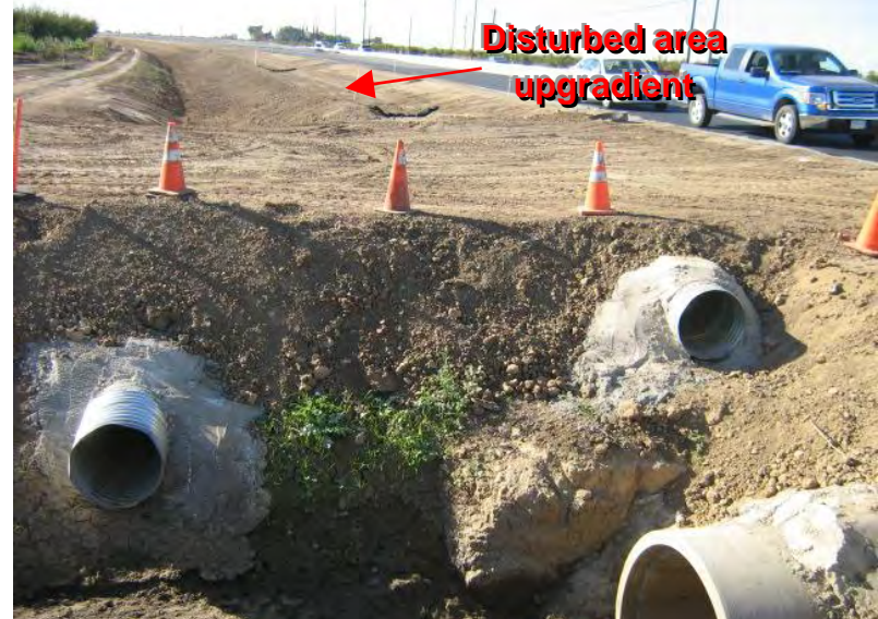
Photograph 6 – Culvert outlet pipes and disturbed embankment slope in irrigation ditch
