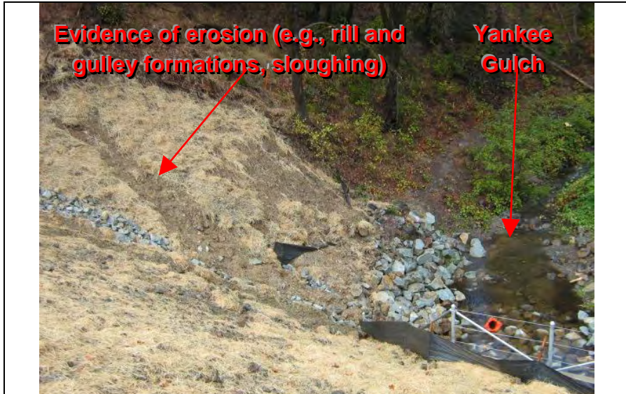
Photograph 9— Evidence of erosion (e.g., rill and gully formation) and sediment transport from the disturbed slope failure
