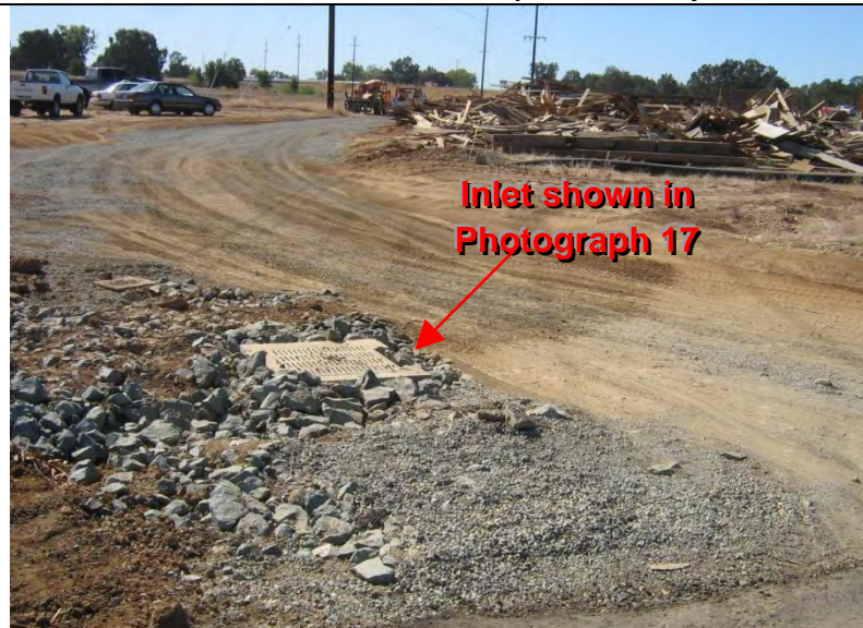
Photographs 16 – Adequate inlet protection and vehicle tracking control BMPs had not been implemented adj. to entrance off Feather River Blvd.
