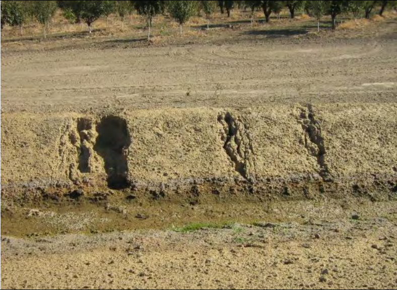
Photograph 17 – Evidence of previous erosion (e.g., rill/gulley formation) was observed on the adjacent roadway drainage swale slopes (West side).
