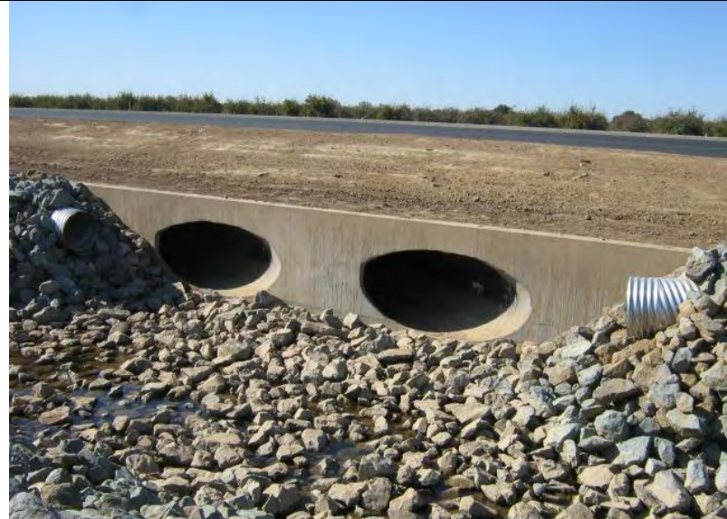
Photograph 14 - Adequate E&S controls were not implemented for areas of disturbance up-gradient of irrigation channel (West side)
