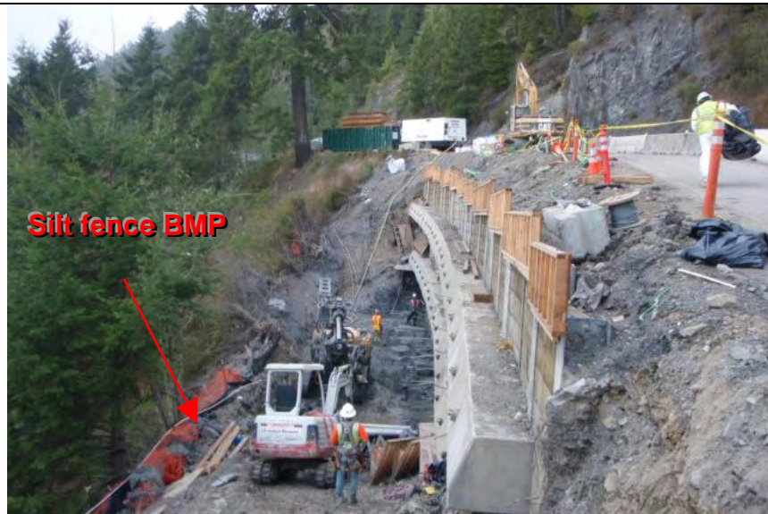
Photograph 2 – Example of silt fence BMP implemented down-gradient of disturbance and retaining wall construction
