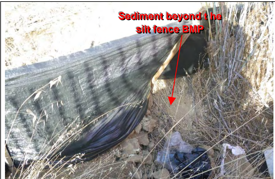
Photograph 5— Failure of first tier of silt fence shown in Photograph 4
