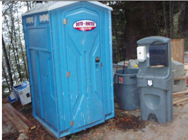
Photograph 12— Portable toilet adjacent to steep slope
