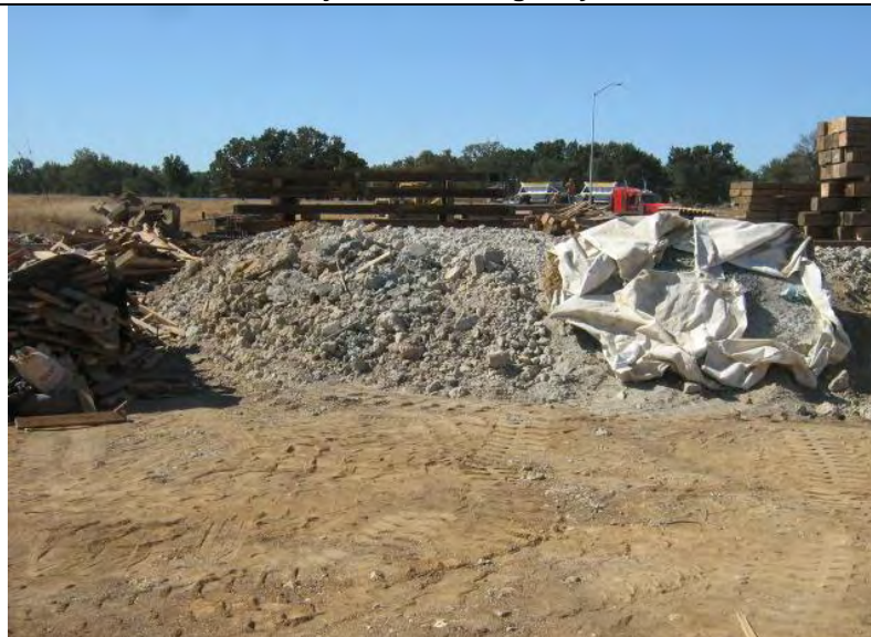
Photograph 8 – Uncontrolled/uncontained concrete waste
