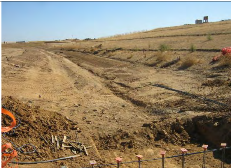
Photograph 8 – Disturbed conveyance channel with no slope run-on BMPs or erosion and sediment control BMPs near the S. Ingram Slough.
