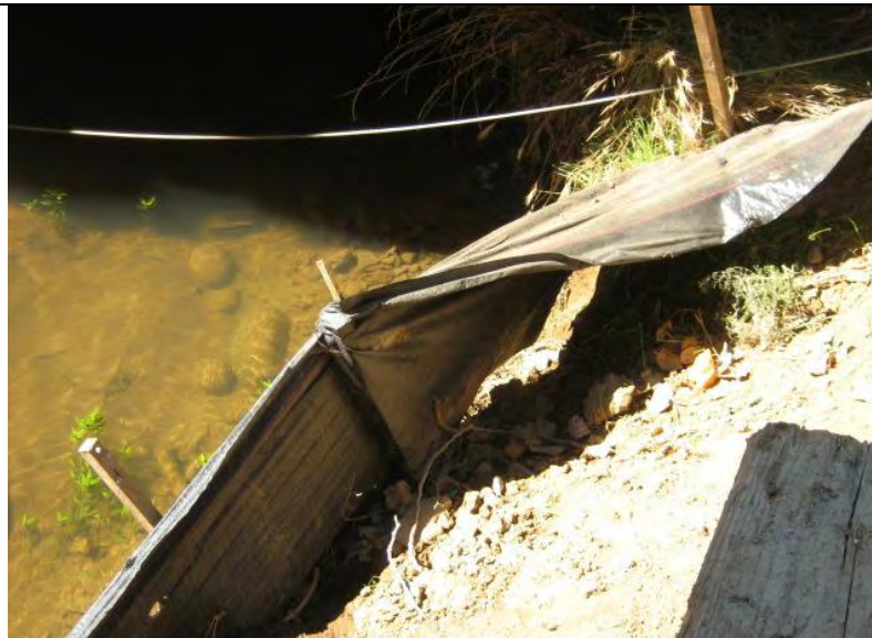
Photograph 24 – Silt Fence not properly entrenched to retain sediment adjacent to Yankee Slough waterway
