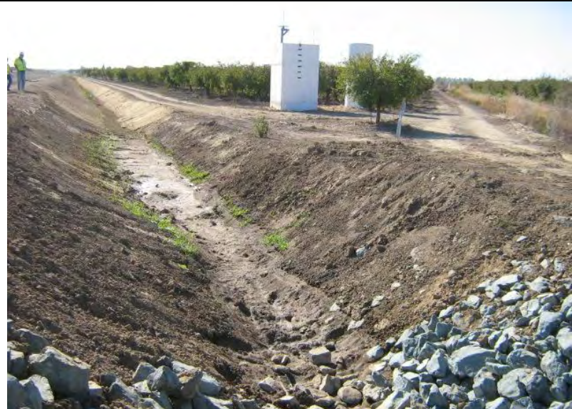
Photographs 16 – BMPs were not implemented for the entire disturbed slope areas of the adjacent roadway drainage swale (East side).
