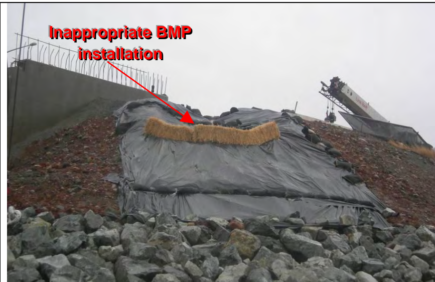
Photograph 1 – View of disturbed slope at Sacramento River Bridge
