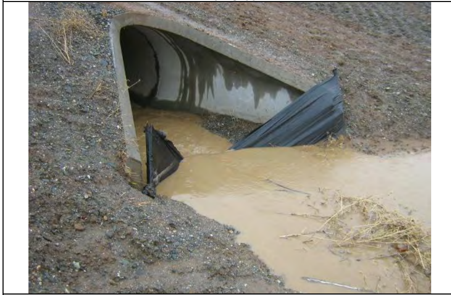
Photograph 11— Collapsed silt fence BMP and discharge of sediment laden runoff
