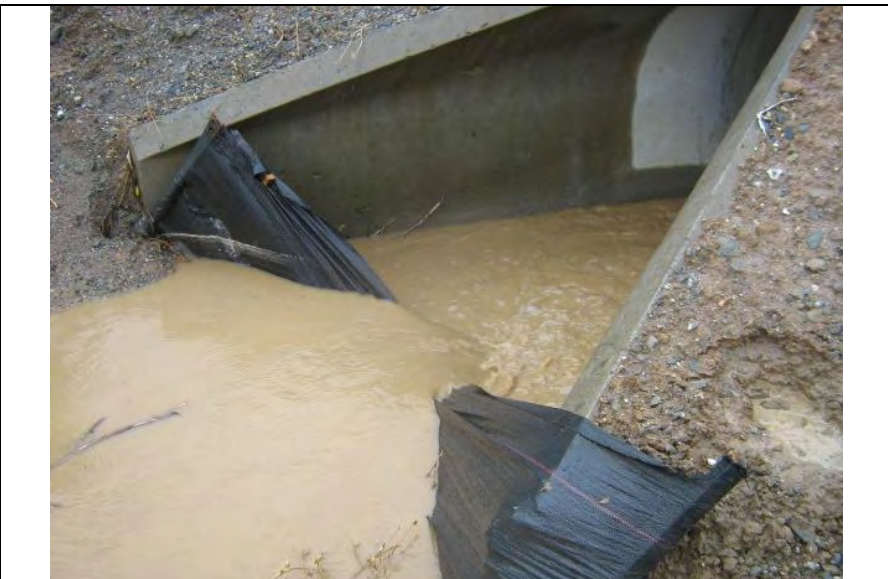
Photograph 10 – Inappropriate BMP selection (e.g., silt fence implemented in area of concentrated flow) and discharge of sediment laden runoff
