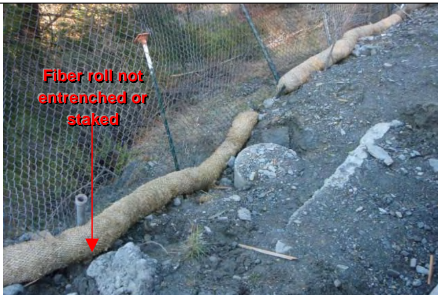
Photograph 3 – Example of fiber roll not entrenched or staked into the ground
