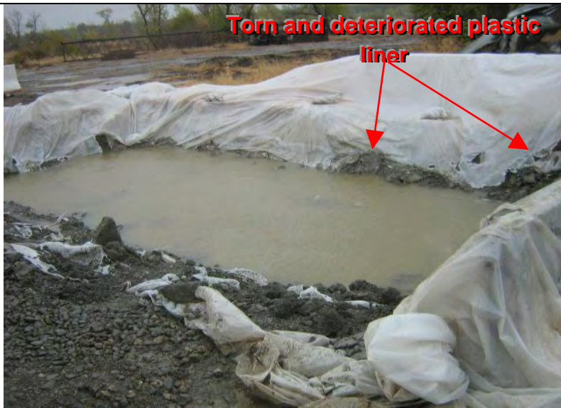
Photograph 1 – Concrete washout unmaintained (e.g., torn and deteriorated plastic liner)
