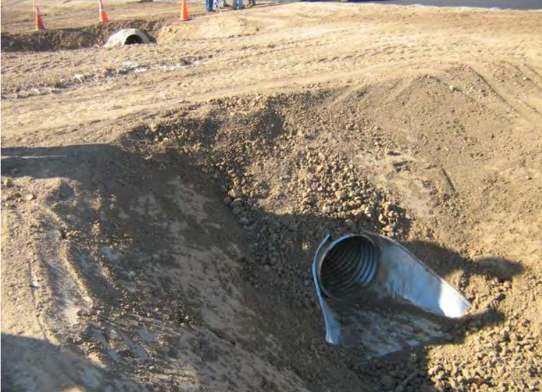
Photograph 7 – Culvert pipe inlet with no BMPs implemented – drains to irrigation ditch.
