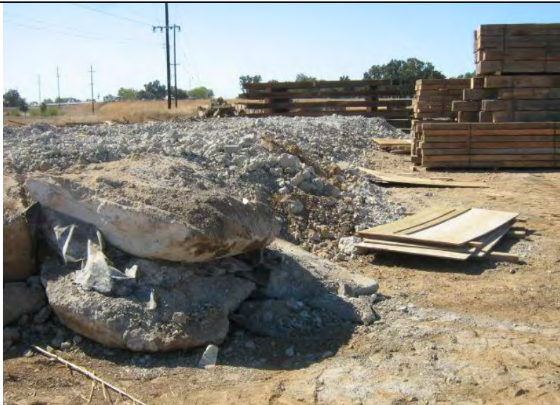
Photograph 9 – Uncontrolled/uncontained concrete waste
