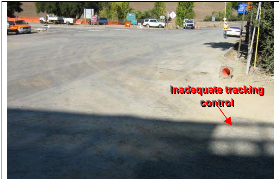
Photograph 9— Sediment conveyed onto roadway
