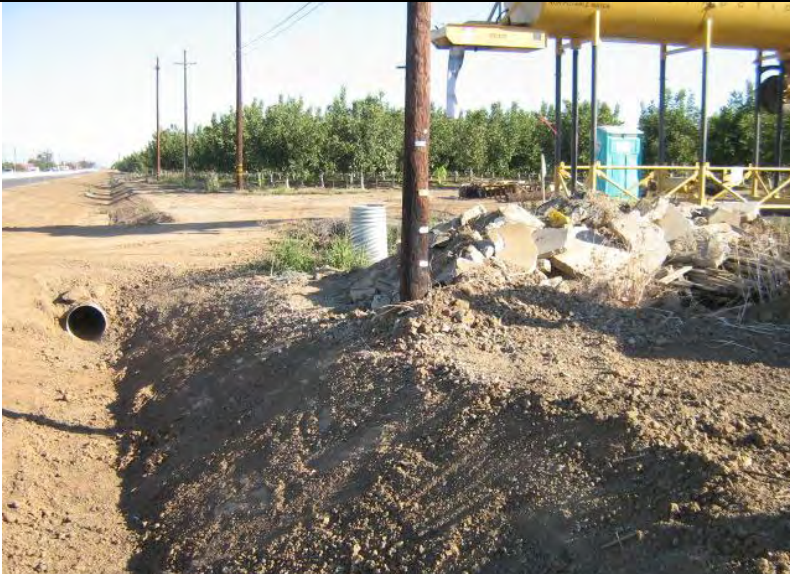
Photograph 3 – Uncontained concrete waste adjacent to roadway drainage swale
