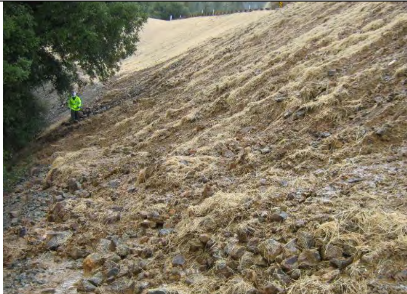
Photograph 2 – Evidence of erosion and slope failure on disturbed slope areas draining to Crystal Creek on the south side of State Highway 299
