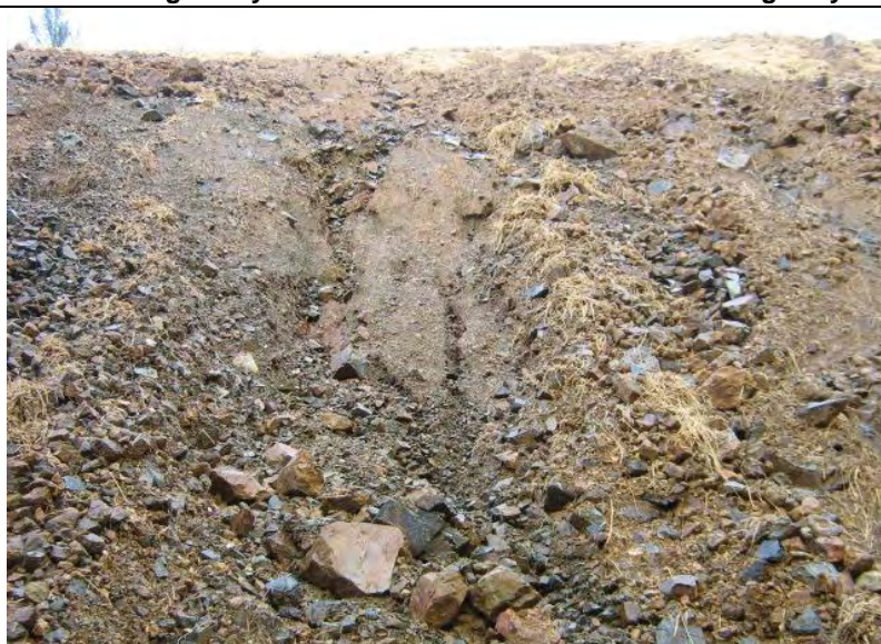
Photograph 4 – Visible evidence of erosion (e.g., rill and gully formation) on the disturbed slope area draining to Crystal Creek
