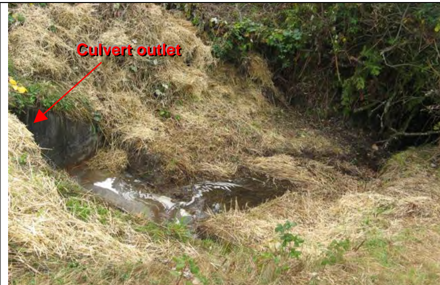
Photograph 6 – West side of culvert outlet (Note: Straw around and within drainage channel)
