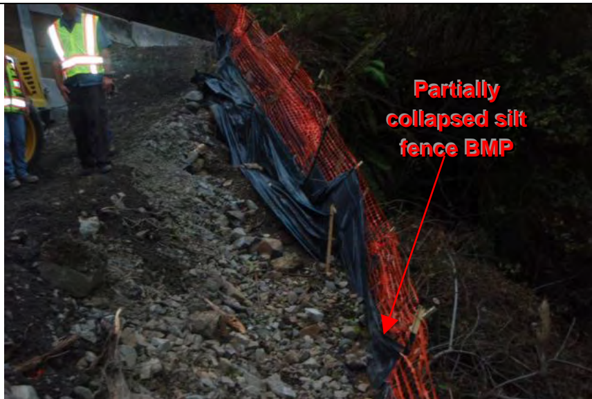
Photograph 5— Another example of sediment accumulation and unmaintained silt fence
