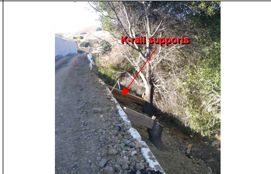
Photograph 4 – Failed area along access road
