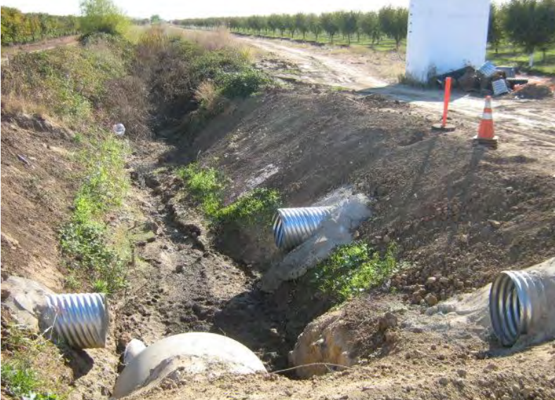
Photograph 5 – View looking upgradient on irrigation channel located adjacent to project. Note unstabilized slopes adj. to irrigation channel.
