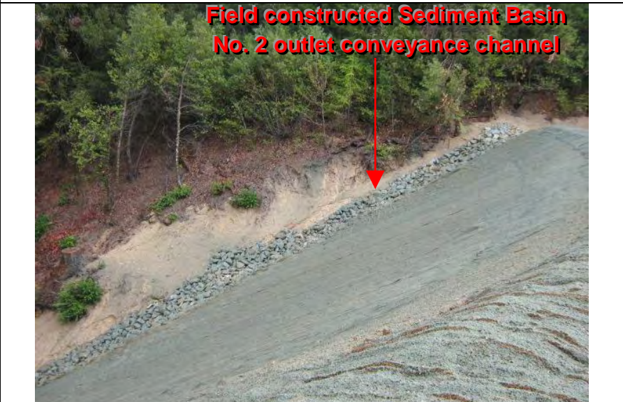
Photograph 4 – Vantage point of the outlet conveyance channel for the field constructed sediment basin No. 2
