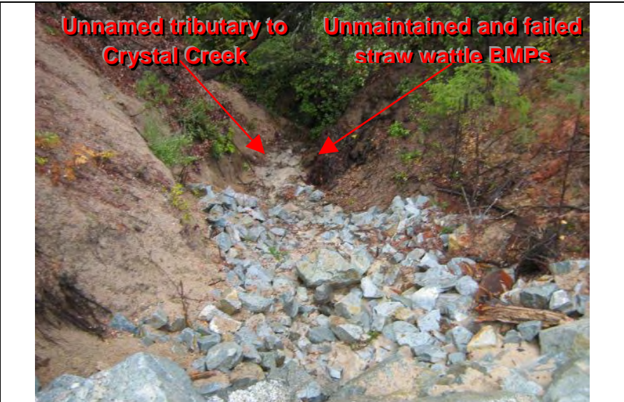
Photograph 6 – Close-up view of sediment basin No. 2 rip-rap outlet conveyance channel to unnamed tributary to Crystal Creek
