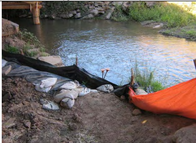
Photograph 12 – Silt Fence BMP not adequately maintained (e.g., down in areas; deteriorated) adjacent to Auburn Ravine
