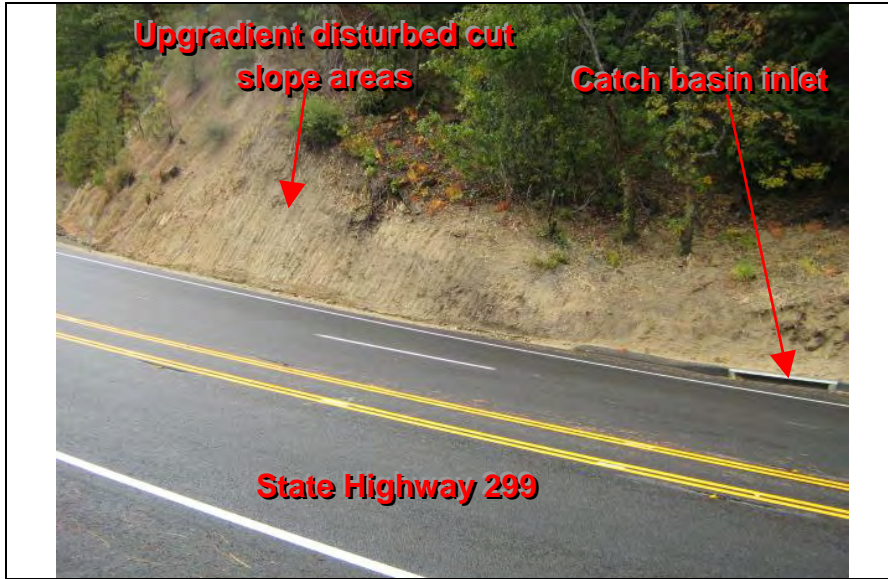
Photograph 21—BMPs were not implemented to prevent the discharge of sediment from up-gradient disturbed cut slope areas to catch basin inlets.
