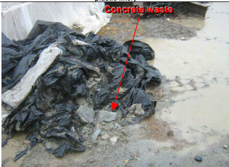
Photograph 3 – Concrete waste on the ground surface directly adjacent to the concrete washout
