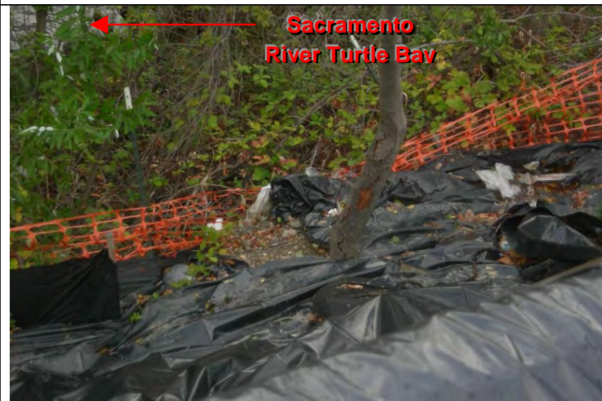
Photograph 3 – View of deteriorated slope stabilization BMP and collapsed silt fence in Photograph 2
