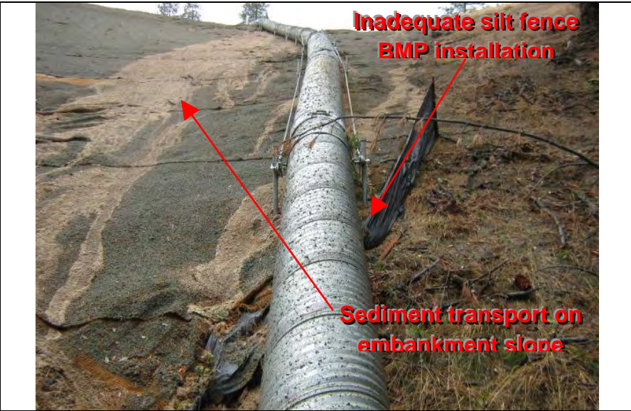
Photograph 14 – Evidence of sediment transport on the embankment slope of the field constructed sediment basin No. 2. Inadequate silt fence BMP installation under culvert pipe
