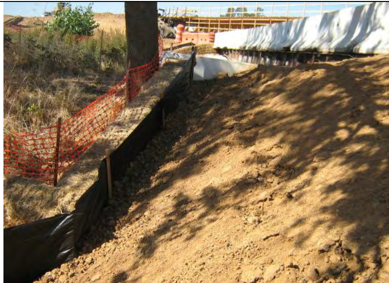
Photograph 10 – Silt fence BMPs installed backwards (e.g., stakes on the upgradient side of the fabric)
