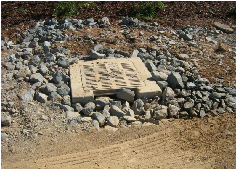
Photograph 17 – Close-up of Photograph 16. Adequate inlet protection had not been implemented.
