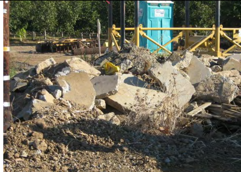
Photograph 4 – Close-up of Photograph 3 and concrete waste
