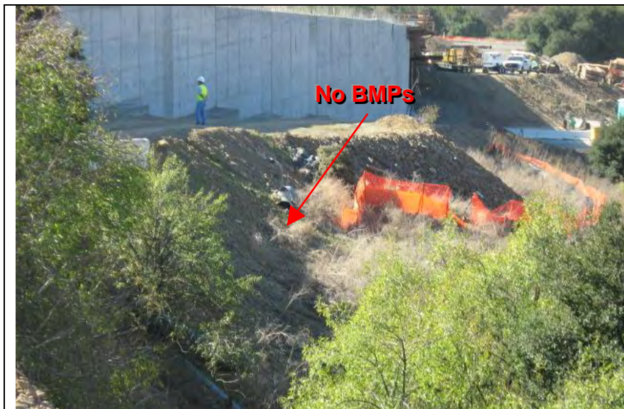
Photograph 5— Fill slope along access road without BMPs
