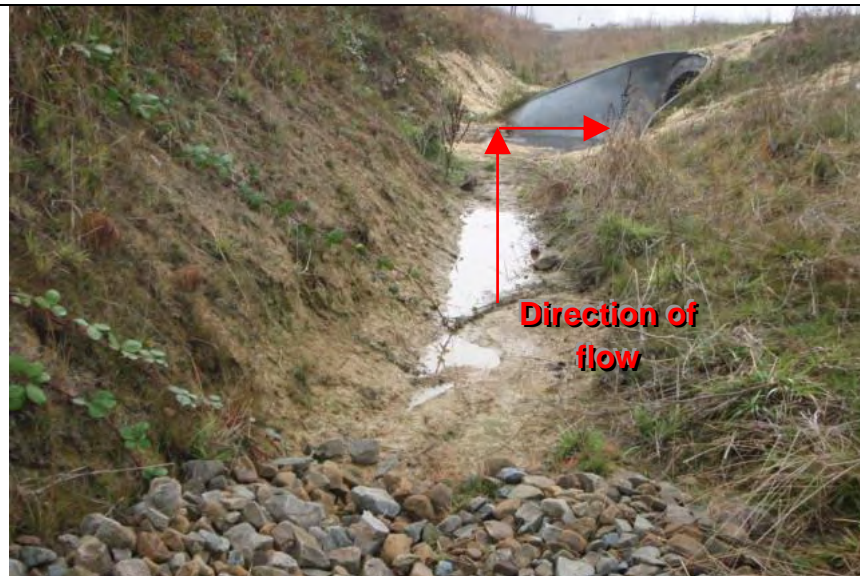
Photograph 2 – Closer view of disturbed drainage ditch and culvert inlet
