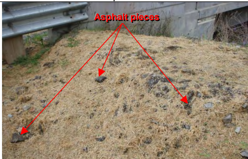
Photograph 11— Sidecast asphalt pieces along side of roadway at northern end of construction project
