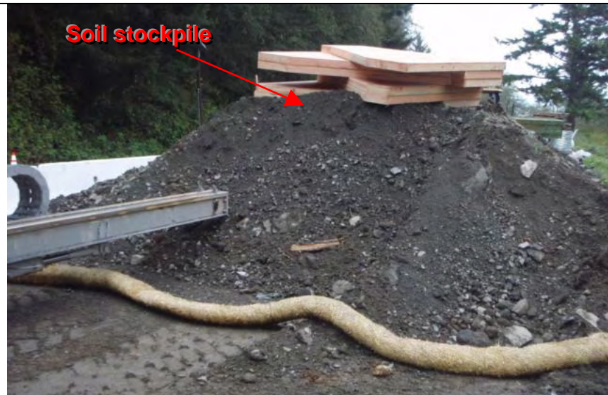
Photograph 14— Another example of straw wattle not staked or entrenched into ground. Inappropriate application of wattles on impervious surface.
