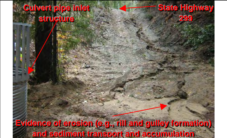
Photographs 20 – Evidence of erosion (e.g. rill and gully formation) and sediment transport from upgradient disturbed slope area (see Photo 18+19)
