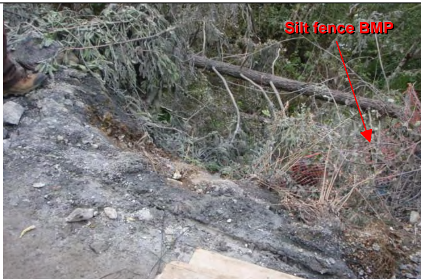
Photograph 7— Another example of silt fence BMP partially covered by collapsed vegetation - view down slope to silt fence BMP
