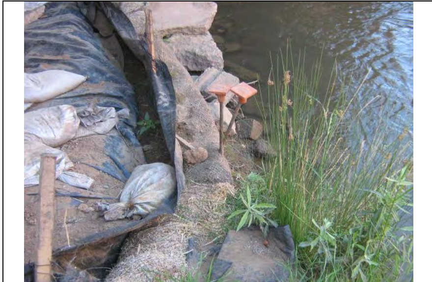
Photograph 13 – Differing vantage point from Photograph 12 depicting unmaintained Silt Fence BMP adjacent to Auburn Ravine
