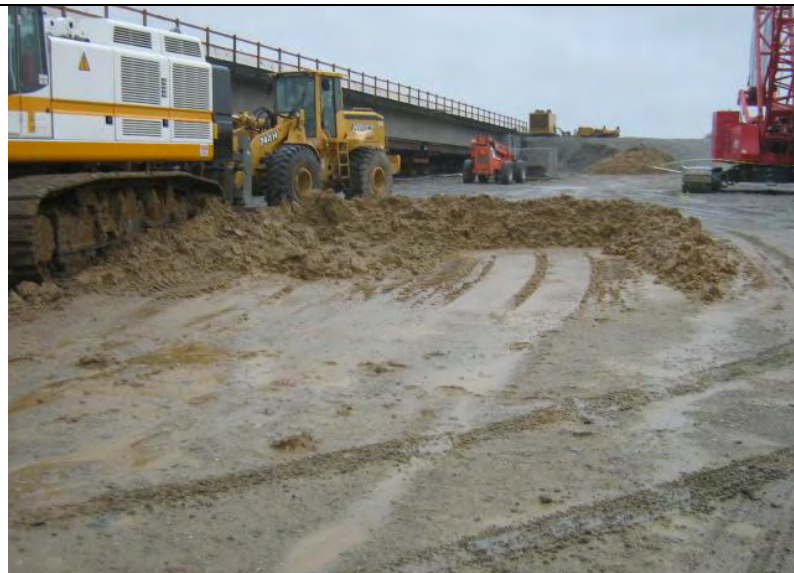
Photograph 10 – Unconsolidated soils without BMPs
