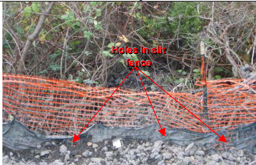
Photograph 4 – Another example of sediment accumulation and unmaintained silt fence
