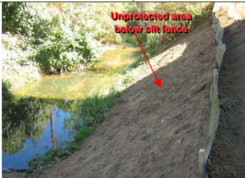
Photograph 19 – Unstabilized slope area adjacent to Yankee Slough
