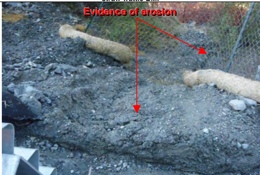
Photograph 7— Undercut section of straw wattle BMP and evidence of erosion
