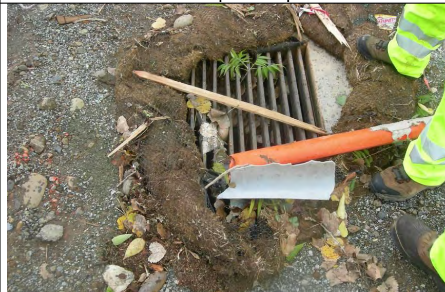
Photograph 7 – Storm drain inlet at the northwestern portion of the Auditorium Drive Bridge temporary staging area
