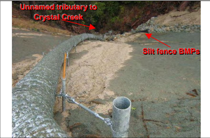
Photograph 13—Adequate BMPs were not implemented to prevent the discharge of sediment from upgradient disturbed slope areas
