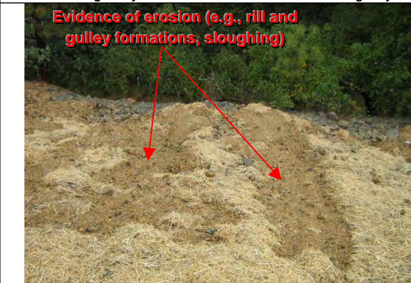
Photograph 3 – Evidence of erosion (e.g., rill and gully formation) and sediment transport from the disturbed slope failure
