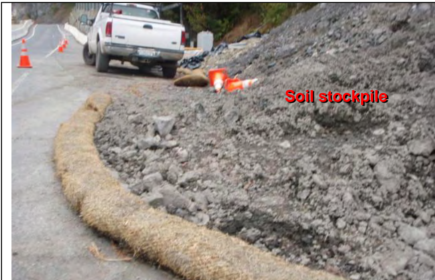
Photograph 13— Straw wattle not staked or entrenched into ground. Inappropriate application of wattles on impervious surface
