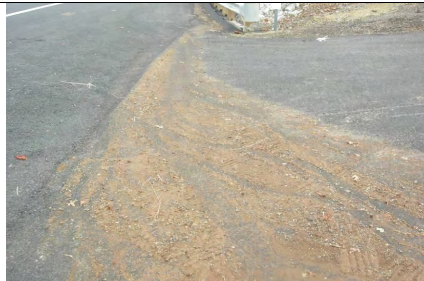
Photograph 6 – Sediment discharge along the highway from Photograph 5
