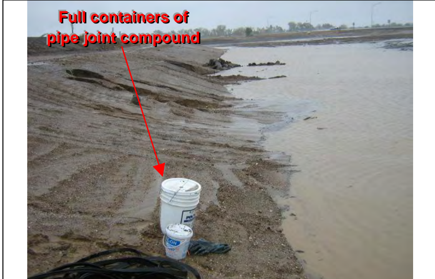
Photograph 7—Pipe joint compound located in the eastern sediment basin
