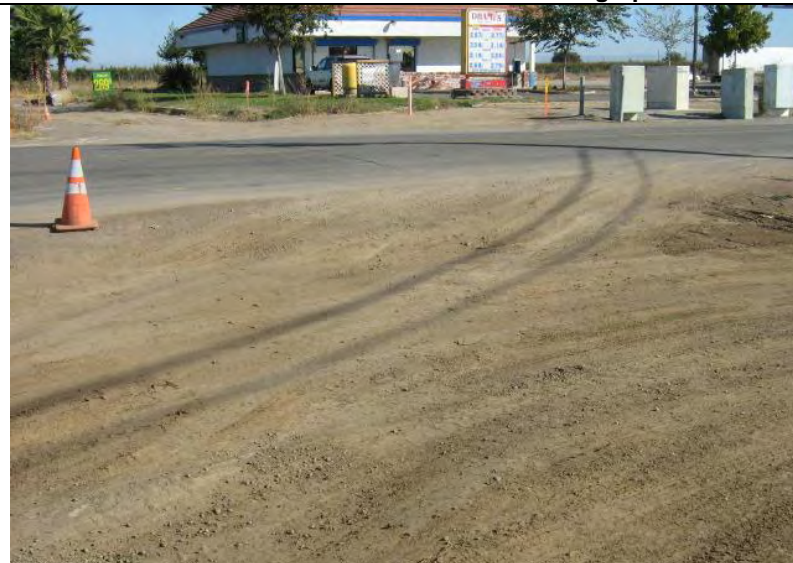
Photograph 12 – No tracking control BMPs implemented at Sta. 346 + 70.
