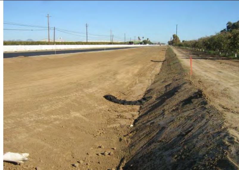
Photograph 2 – Unstabilized drainage swale and slope adjacent to roadway
