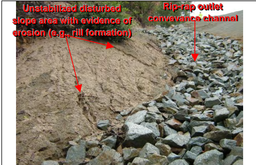
Photograph 17—Adequate BMPs were not implemented to prevent the discharge of sediment from disturbed slope area adjacent to the rip-rap conveyance channel which drains to the unnamed tributary.
