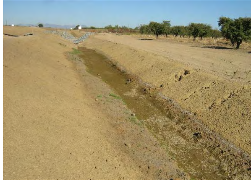
Photograph 18 – Vantage point view of Photograph 17. Adjacent roadway swale drains to irrigation channel near top of Photograph.
