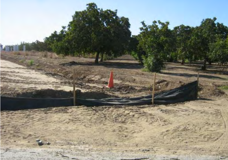
Photograph 19 – Silt fence not adequately maintained (e.g., collapsed in areas) near the new Hwy 99 and Wilson Road intersection.
