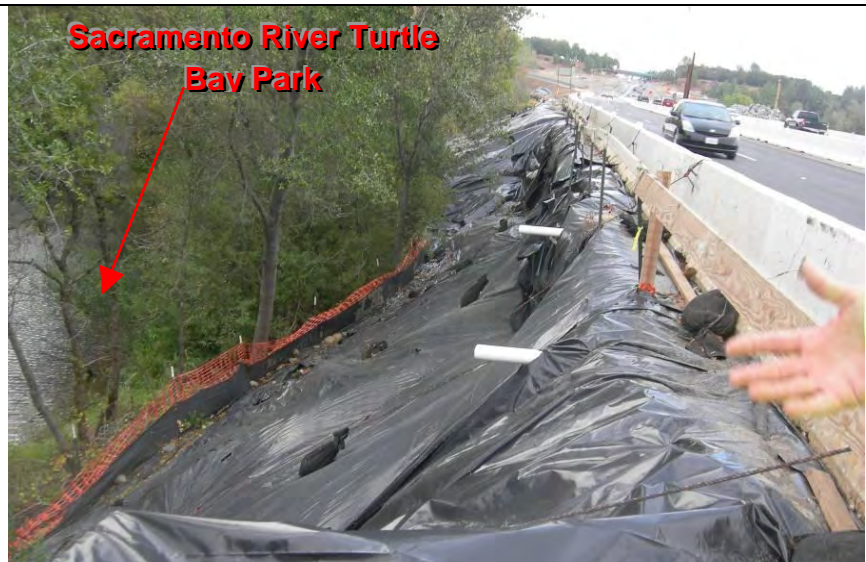
Photograph 2 – View of temporary plastic slope stabilization along the north side of I-5, at the terminus of the bike path
