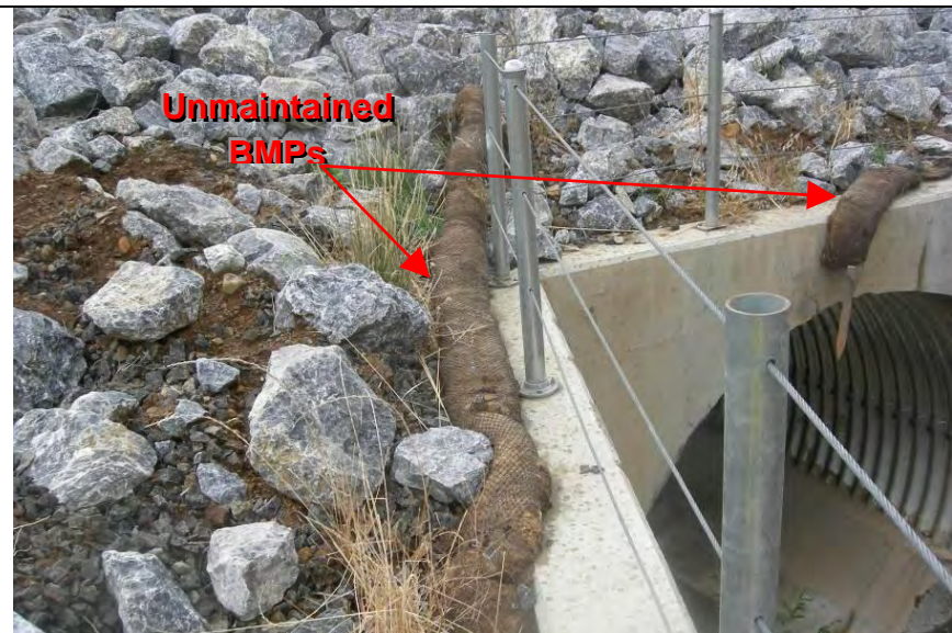
Photograph 8 – Inadequate straw wattle BMP maintenance at drainage pipe inlet
