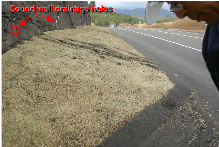
Photograph 2 – Run-off causing erosion along the highway shoulder
