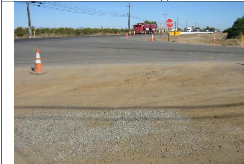
Photograph 11 –Tracking control BMPs were not implemented near Station 346 + 70.
