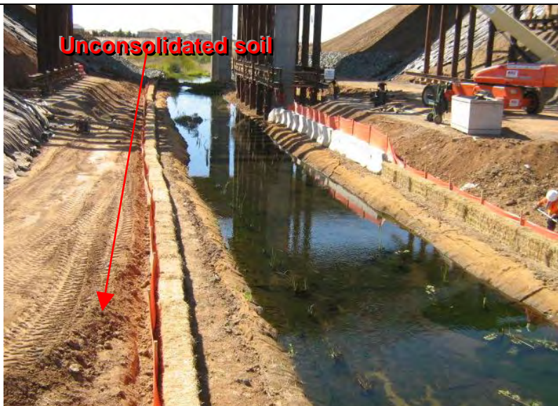
Photograph 3 – Unconsolidated soil placed between the toe of the slope and the perimeter control BMPs along the waterway
