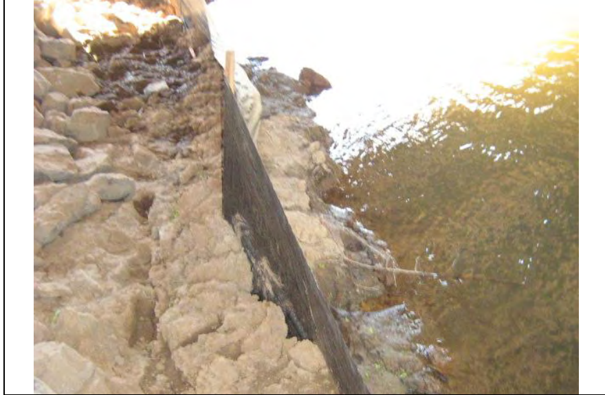
Photograph 15 – SF BMP not adequately maintained (e.g., sediment placement over ½ the effective height) adjacent to Auburn Ravine
