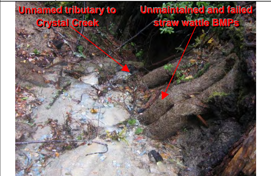
Photograph 8 – Visible evidence of the discharge of sediment to the unnamed tributary to Crystal Creek, and failed straw wattle BMPs observed
