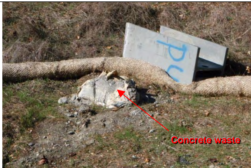
Photograph 11— Concrete waste near concrete waste container in staging area (Note: Straw wattle BMP not staked or entrenched into ground)
