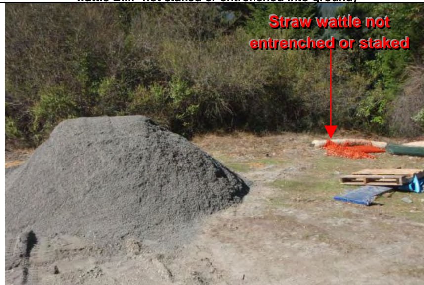
Photograph 12— Stockpile in staging area without BMPs for containment or coverage
