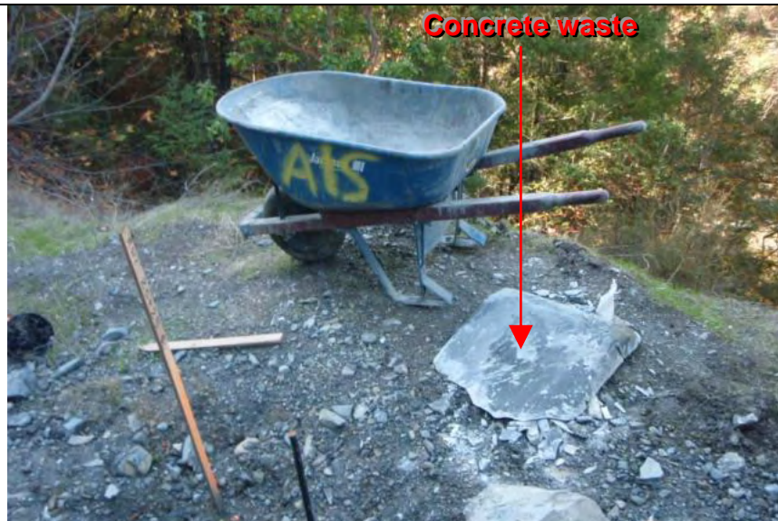
Photograph 9— Concrete waste on ground surface adjacent to steep slope
