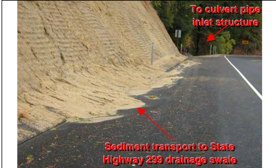
Photograph 19—Evidence of sediment transport to State Highway 299 drainage swale from the adjacent unstabilized disturbed cut slope area.
