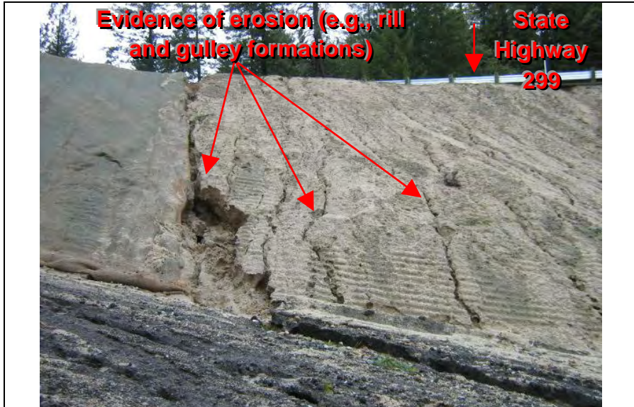
Photograph 1 – Disturbed slope areas adjacent to State Highway 299 with evidence of erosion (e.g., rill and gully formations)
