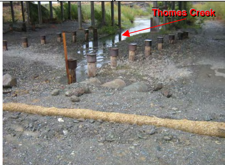
Photograph 8 – Erosion log BMPs were not adequately installed (e.g., not properly staked) adjacent to the flowing Thomes Creek
