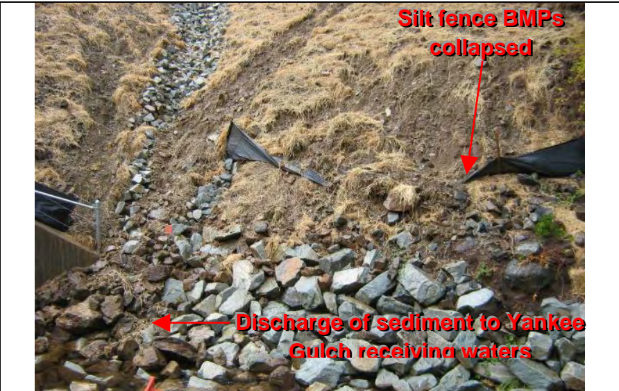
Photograph 10 – Silt fence BMPs collapsed in areas and evidence of the discharge of sediment to Yankee Gulch
