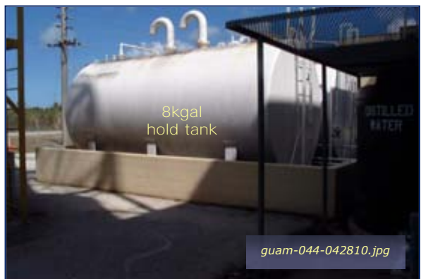
Photo #4-24: Bldg 307 Orote Power Plant - 8K Hold Tank Taken By: Greg V. Arthur Date: 04/28/10
