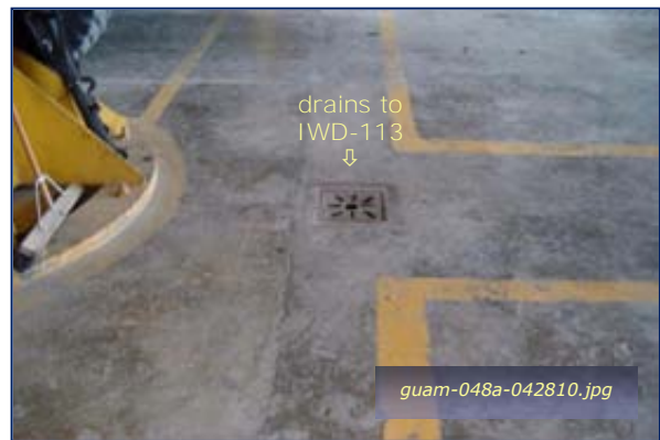
Photo #4-32: Bldg 557C - Example Floor Drain Taken By: Greg V. Arthur Date: 04/28/10
