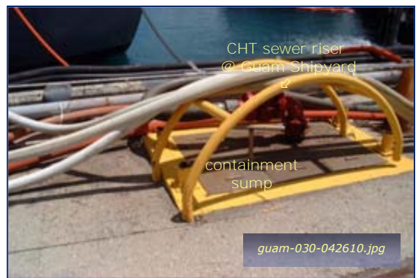
Photo #3-8: November Wharf CHT Sewer Riser Taken By: Greg V. Arthur Date: 04/26/10
