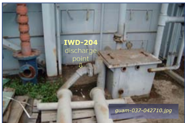
Photo #5-6: Bldg 27 Paint Shop - Sewer Connection Taken By: Greg V. Arthur Date: 04/27/10
