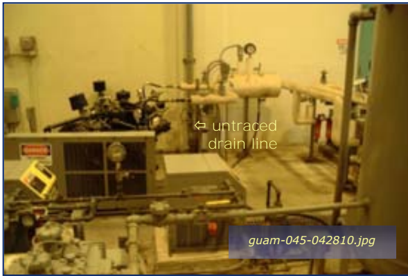
Photo #4-25: Bldg 307 Orote Power Plant - Drain Taken By: Greg V. Arthur Date: 04/28/10
