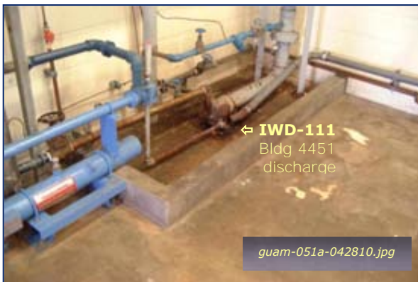
Photo #4-29: Bldg 4451 Steam Plant - Boiler Line 1 Taken By: Greg V. Arthur Date: 04/28/10
