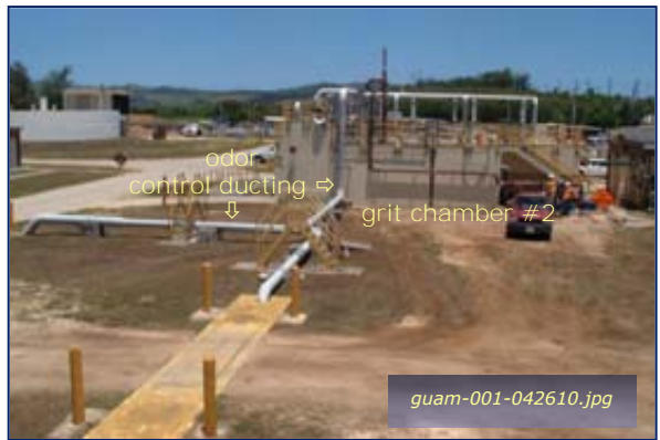
Photo #3-4: Odor Control Duct Lines Taken By: Greg V. Arthur Date: 04/26/10
