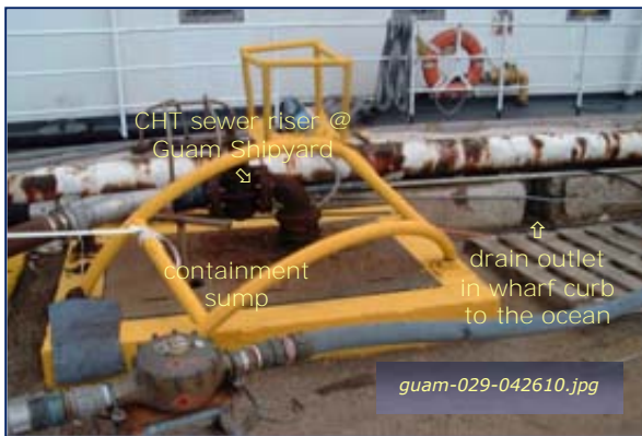
Photo #3-7: Oscar Wharf CHT Sewer Riser Taken By: Greg V. Arthur Date: 04/26/10
