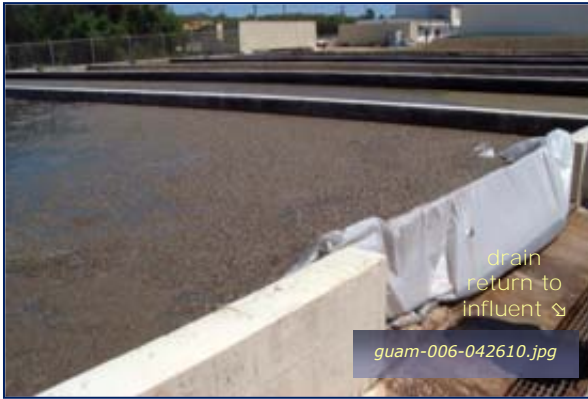
Photo #3-5: Apra Harbor WWTP - Sludge Drying Taken By: Greg V. Arthur Date: 04/26/10
