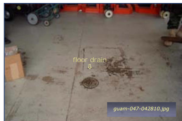
Photo #4-36: Bldg 2113 EOD - Example Floor Drain Taken By: Greg V. Arthur Date: 04/28/10
