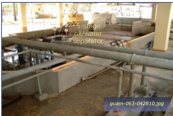
Photo #4-11: FISC Fuel Farm - O/W Gravity Sep Taken By: Greg V. Arthur Date: 04/28/10
