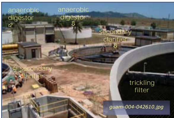
Photo #3-3: Secondary Clarifiers and Digestors Taken By: Greg V. Arthur Date: 04/26/10
