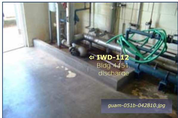
Photo #4-30: Bldg 4451 Steam Plant - Boiler Line 2 Taken By: Greg V. Arthur Date: 04/28/10
