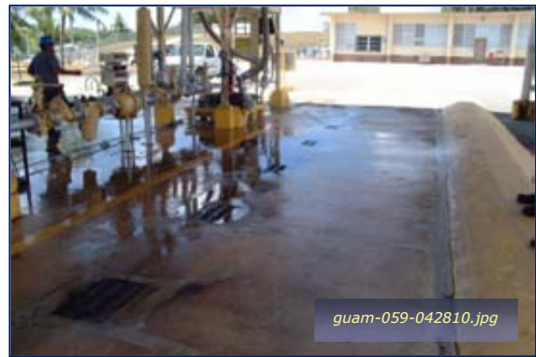
Photo #4-14: FISC Fuel Farm – Bottom Fill Drains Taken By: Greg V. Arthur Date: 04/28/10
