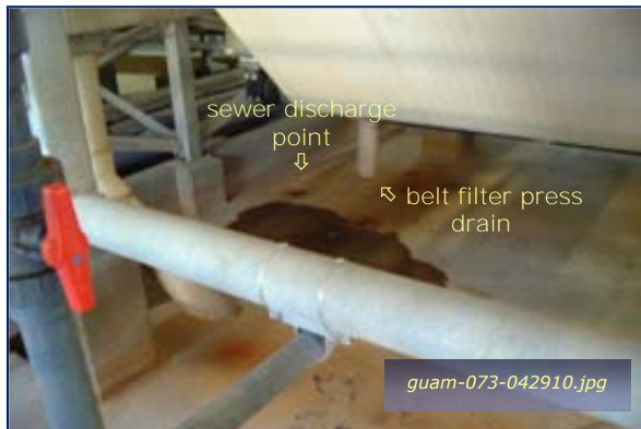
Photo #4-17: Fena WTP – Belt Filtrate Discharge Taken By: Greg V. Arthur Date: 04/29/10
