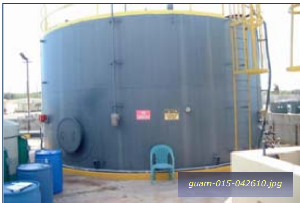
Photo #4-3: Victor Wharf BOWTS – 50kgal EQ Tank Taken By: Greg V. Arthur Date: 04/26/10
