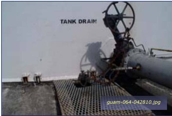
Photo #4-13: FISC Fuel Farm – Tank Bottom Draw Taken By: Greg V. Arthur Date: 04/28/10
