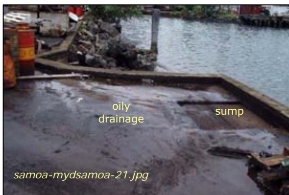
Photo #11: Catch Basin #1 - Discharge Sump 001 Taken By: Greg V. Arthur Date: 04/01/08
