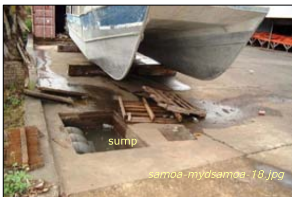
Photo #9: Catch Basin #2 - Discharge Sump 002 Taken By: Greg V. Arthur Date: 04/01/08
