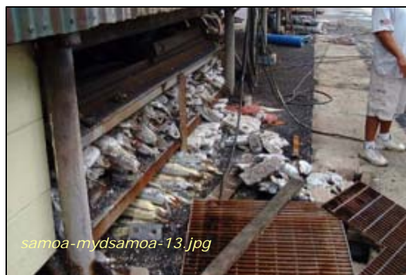
Photo #6: Catch Basin #3 - Zinc Anodes Exposed Taken By: Greg V. Arthur Date: 04/01/08
