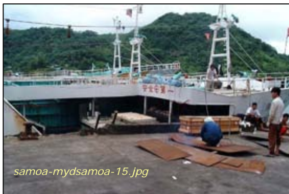
Photo #7: Catch Basin #3 - South Dock Crew Work Taken By: Greg V. Arthur Date: 04/01/08
