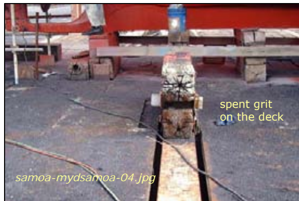
Photo #2: 3000-Ton Dry Dock - Gaps in Decking Taken By: Greg V. Arthur Date: 04/01/08
