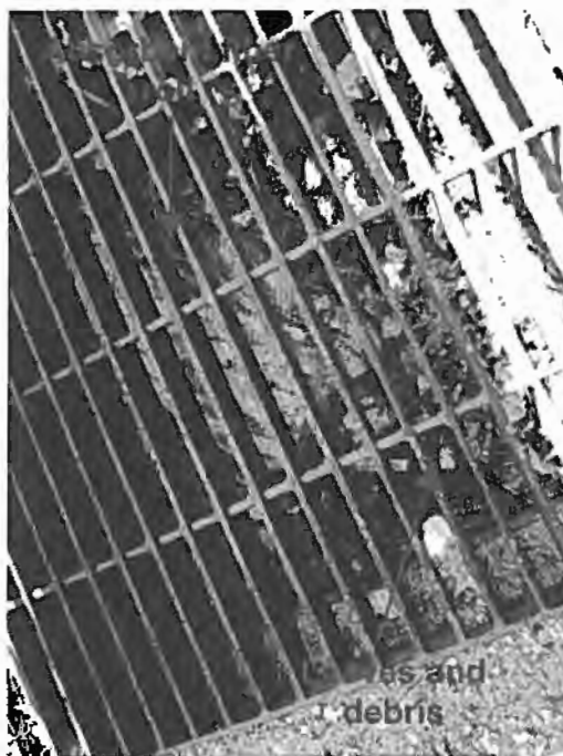
Photograph 6. Bill's Quality Auto Care – Close-up view inside the storm drain inlet shown in Photograph 5. Note that an absorbent fiber roll BMP had been placed in a drain to prevent further conveyance of petroleum to the site outfall. In addition there were leaves and debris within the catch basin.
