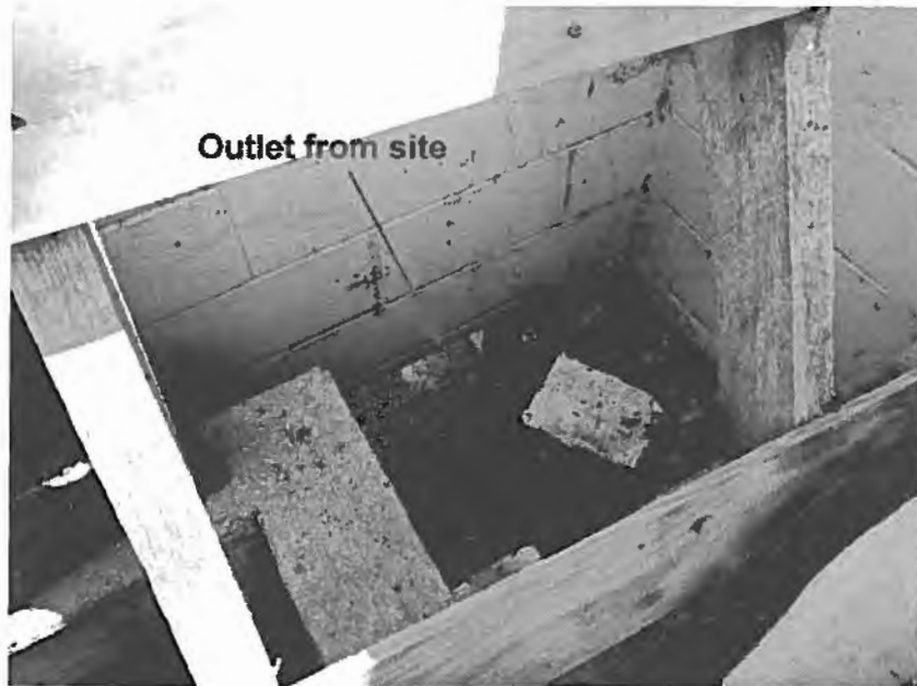
Photograph 7. Bill's Quality Auto Care – View of an outlet from the site located in the southeast corner of the facility.
