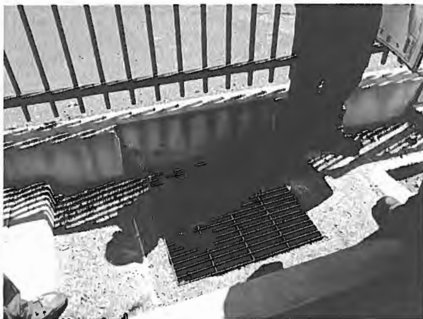
Photograph 5. Bill's Quality Auto Care – View of a storm drain inlet located on the south side of the facility yard.
