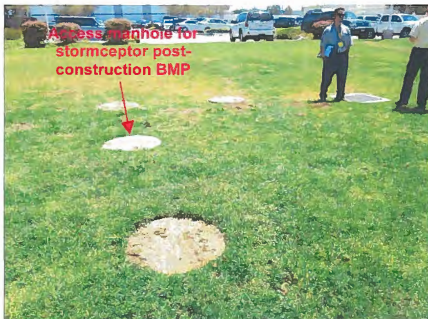
Photograph 5. PTI Facility I/C Site Visit – View of access manhole for stormceptor located on the north end of the facility.
