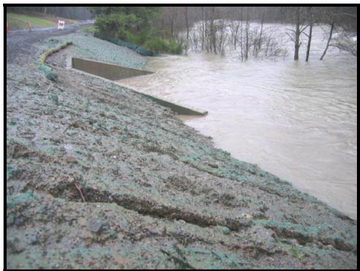
Photograph 2. Lower Mad Road (insloped and paved) looking east during December 2005 flood event. Surface runoff from road causing gully erosion on road fill and directly delivering sediment to the Mad River. Note silt fence completely inundated in background.
