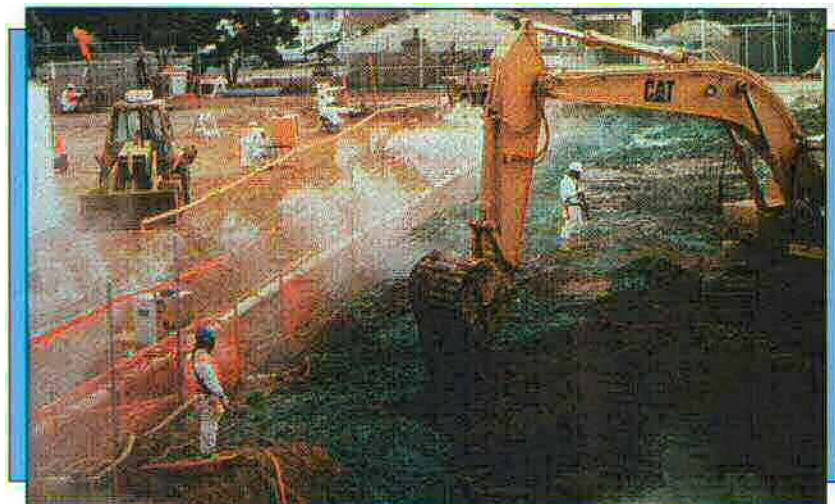
A very dilute ODEX solution is shown atomized around the perimeter of a large Superfund site to eliminate odors. HydroSeal was also used. During the 13 months KUMA was on site, there were no odor-induced shutdowns.
