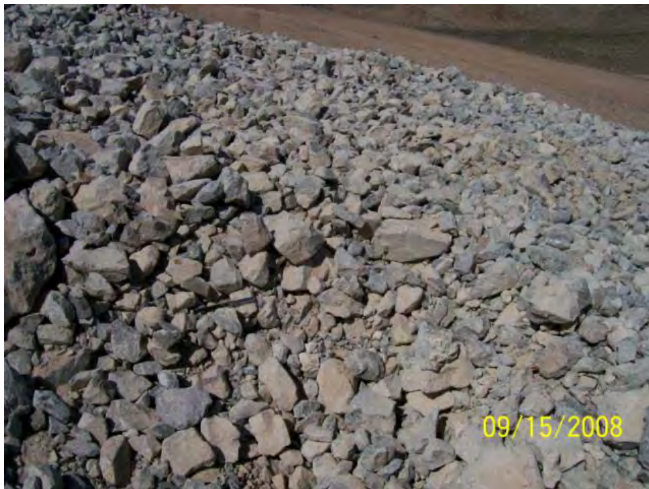
Photo 5 Sidewall of Trench Cut through Erosion Layer. Note the Well Graded Matrix
