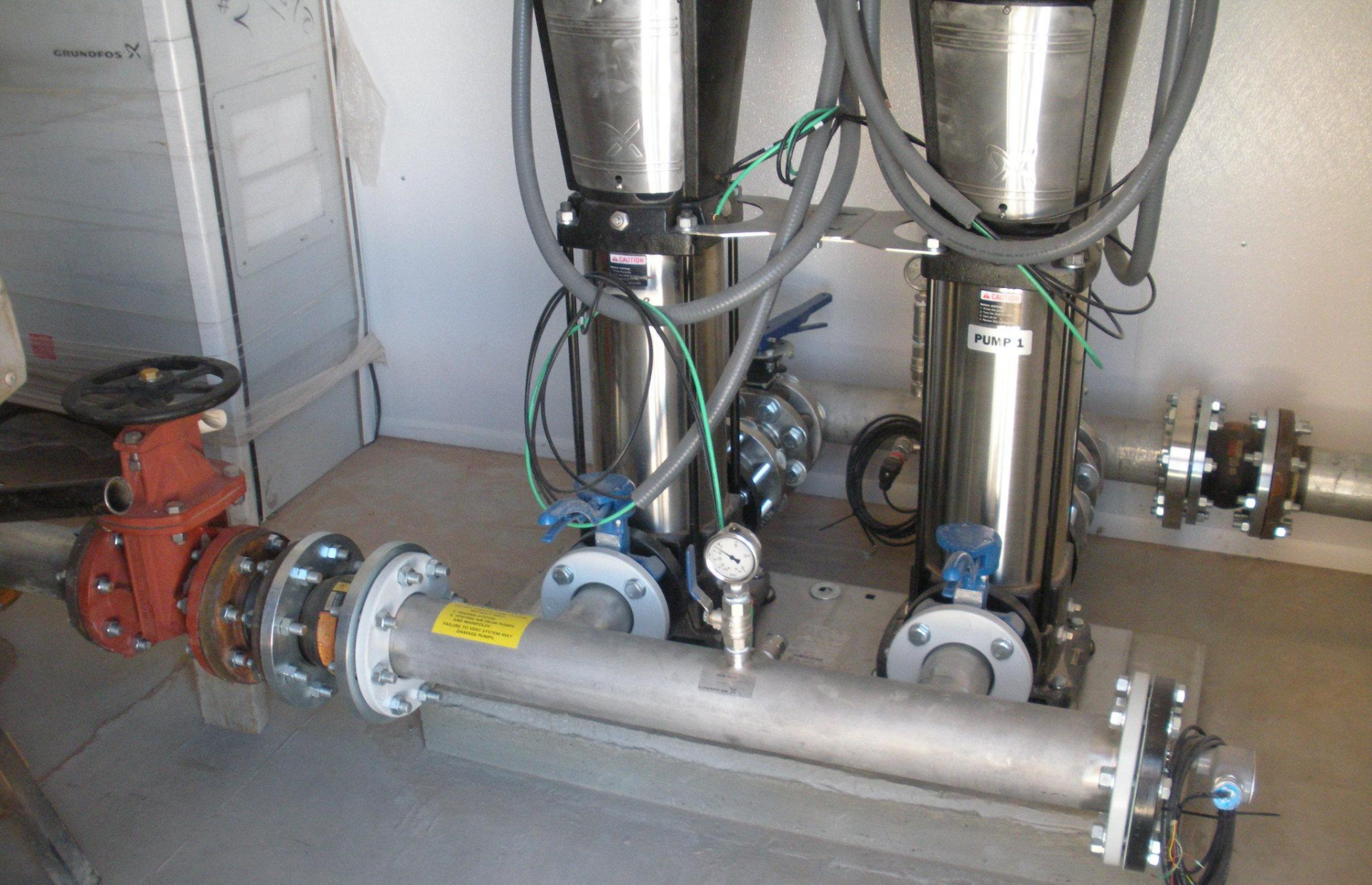
Sweetwater Booster Pumps
