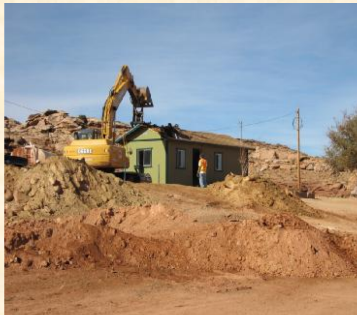
House built on mill tailings
