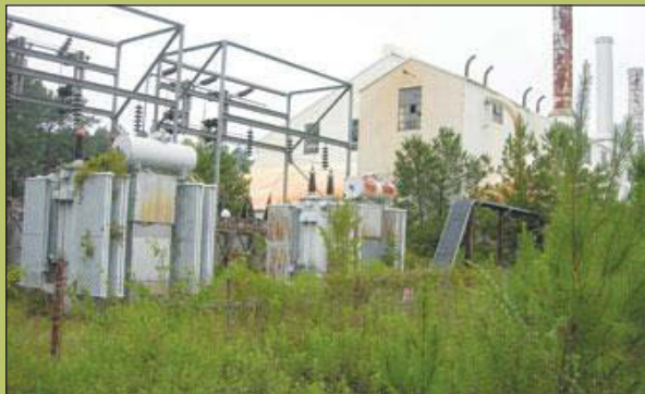
PICTURED: Abandoned powerhouse facility on LHAAP property. (source: Marshall News Messenger)
