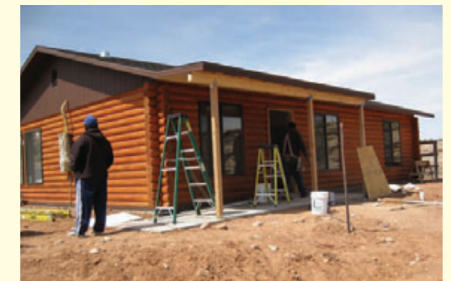
Replacement structure in Red Valley built by majority Navajo-owned company with energy efficiency improvements
