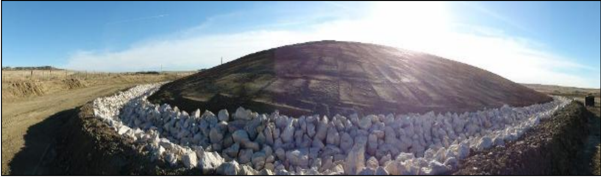
Repository Cell at Section 32/33
