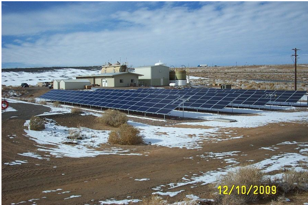
Figure 9: Solar panels at the Tuba City Disposal Cell
