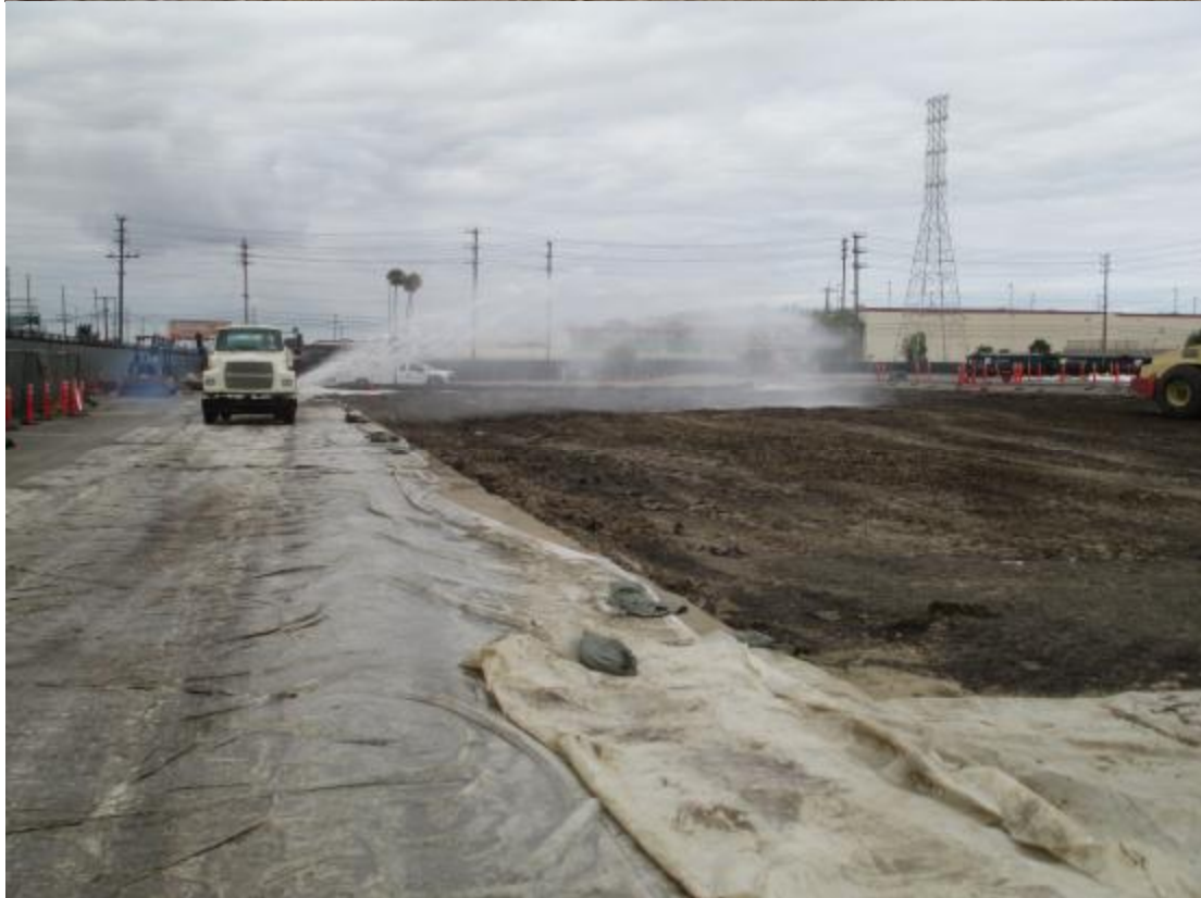
Figure 3: Sheep's foot dynamic compactor working fill (top) and water truck spraying fill (bottom).
