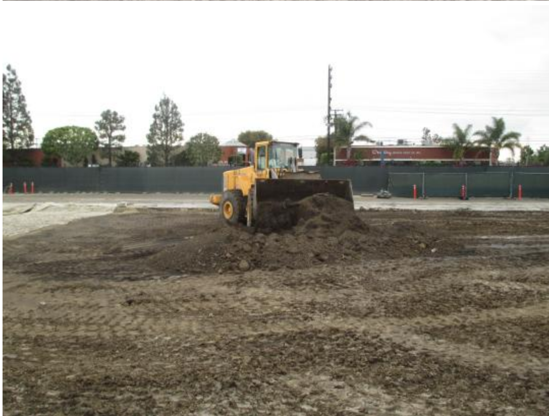
Figure 1: crushed asphalt and soil piles ready for mixing (top). Asphalt and soil being mixed by front loader, and well blended prior to being placed in fill layers (bottom).
