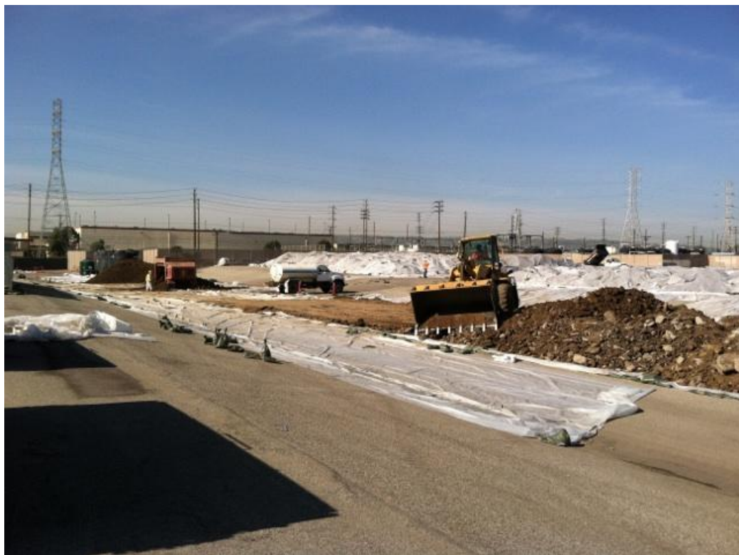
Figure 1: Soil screening - stockpile from excavation north of shaker, shaker (red machine), and stockpile of screened soil south of shaker (distance).
