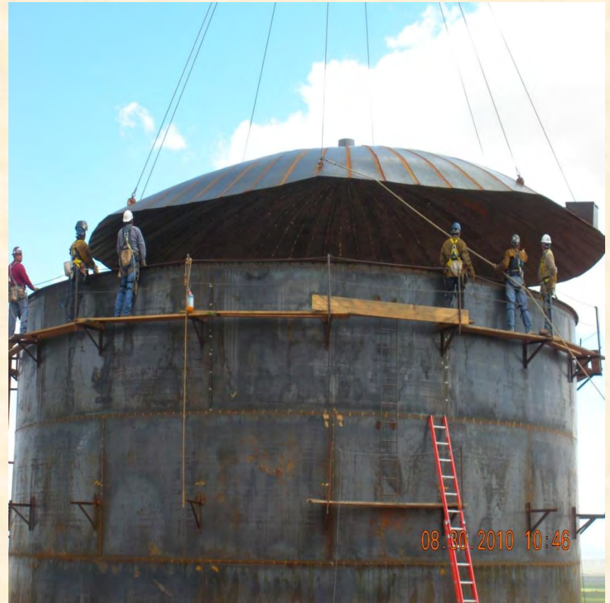
Sweetwater 500,000 gallon water tank
