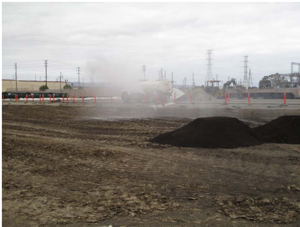
Figure 1: Water truck spraying fill pad to keep the soils conditioned for placement as engineered fill and for dust control. No dust observed.
