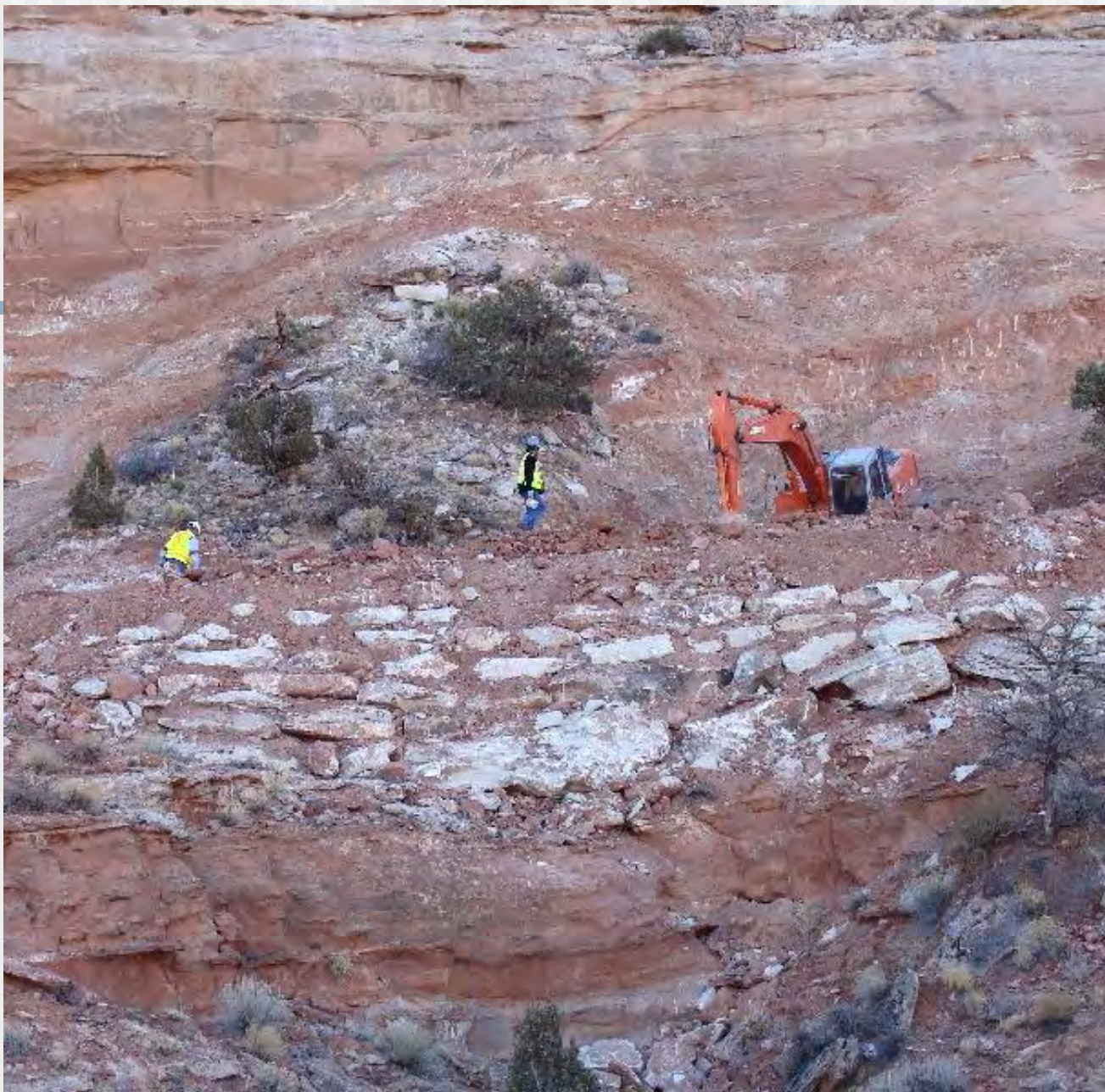
Inaccessible mine waste and contained.
