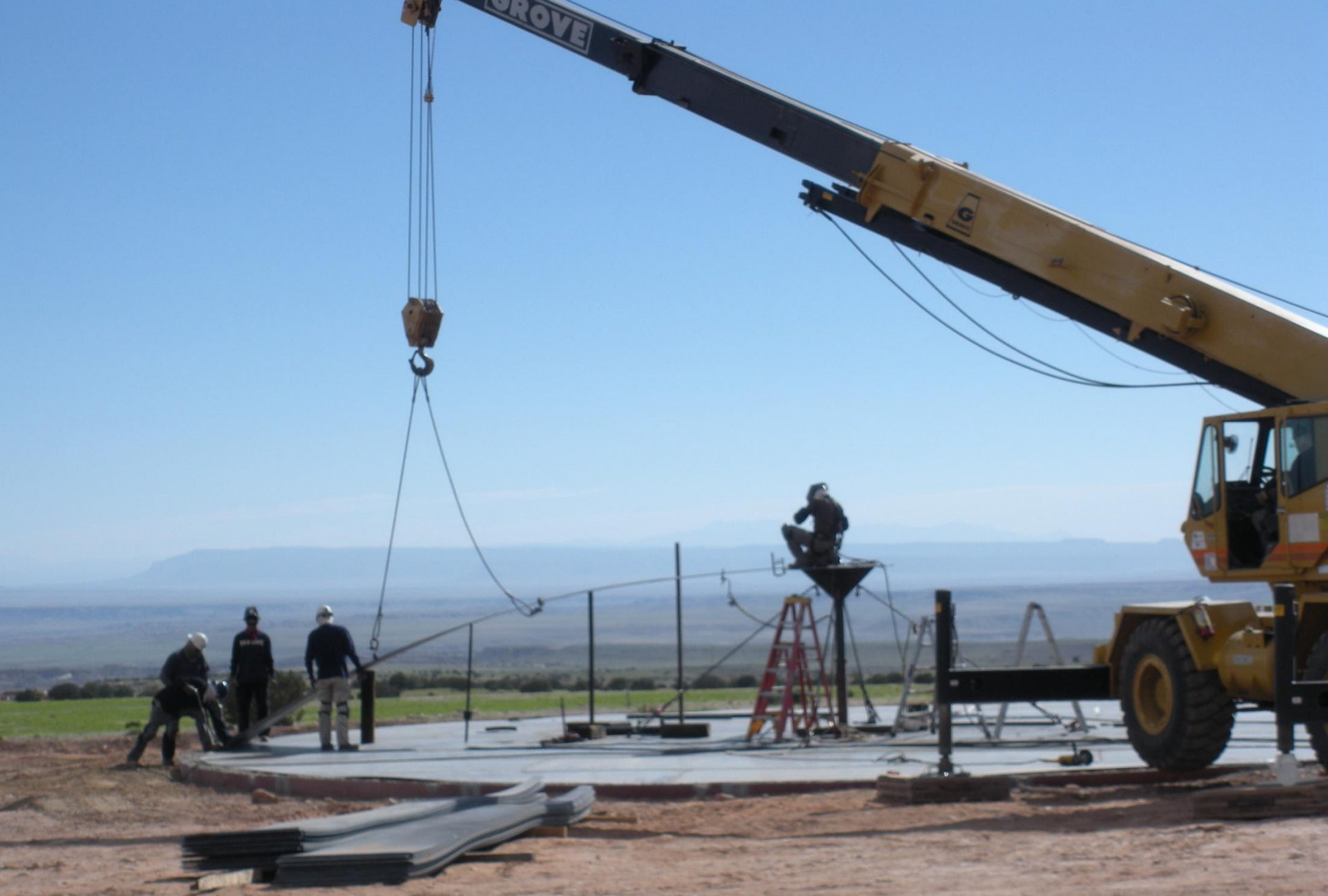
500,000 gallon water storage tank in Teec Nos Pos
