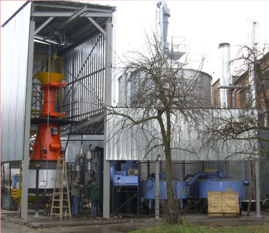
Downdraft Gasifier similar to the Los Banos project
