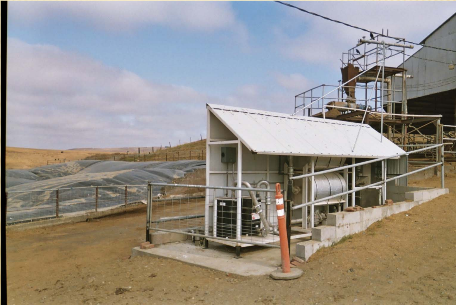
Carbon Canister Hydrogen Sulfide Removal, Refrigerated Gas drier and blower
