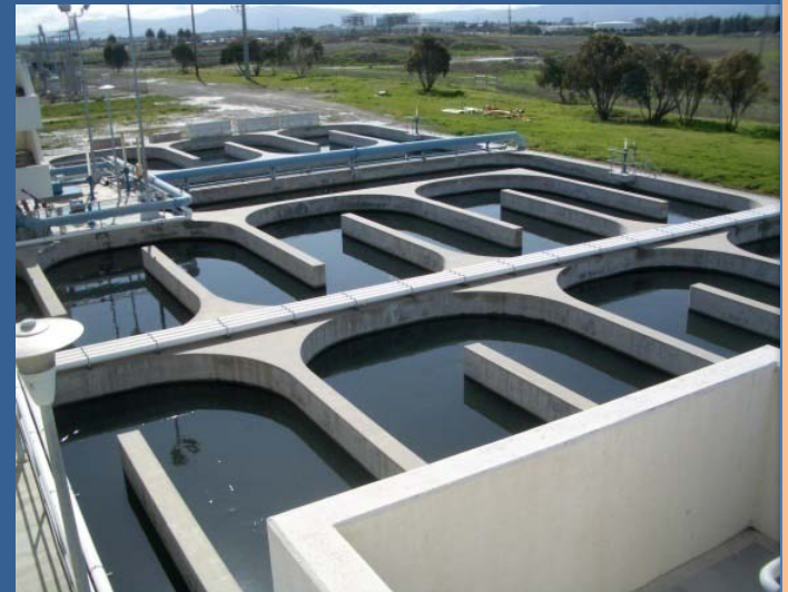
Photo: J. Franco – City of San Jose WWTP
