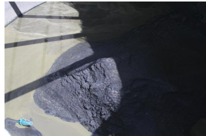
Sand in Digester
