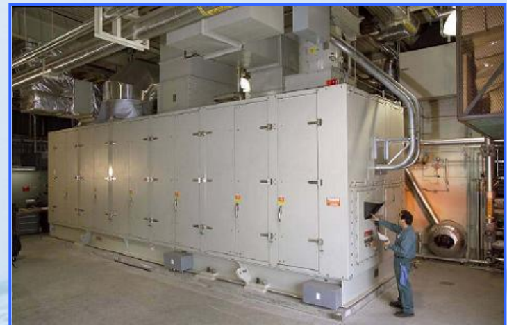
3.5 MW gas turbine Cogeneration System
