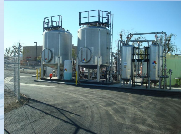
Digester Gas Treatment System, EMWD-Moreno Valley, CA
