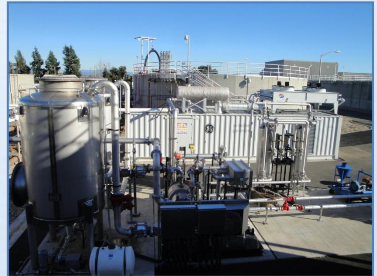
335-kW Digester Gas Fueled Cogeneration System, Chico, CA WWTP
