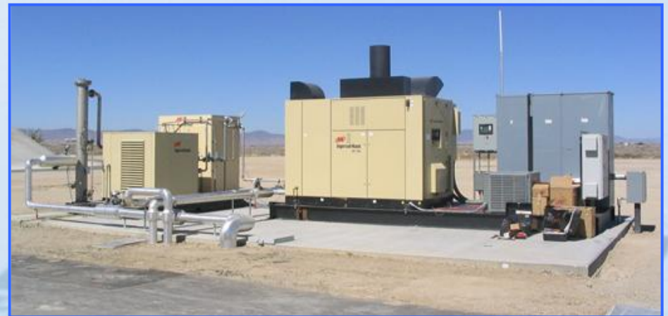
250-kW Landfill Gas Fueled microturbine Cogeneration System, Lancaster, CA
