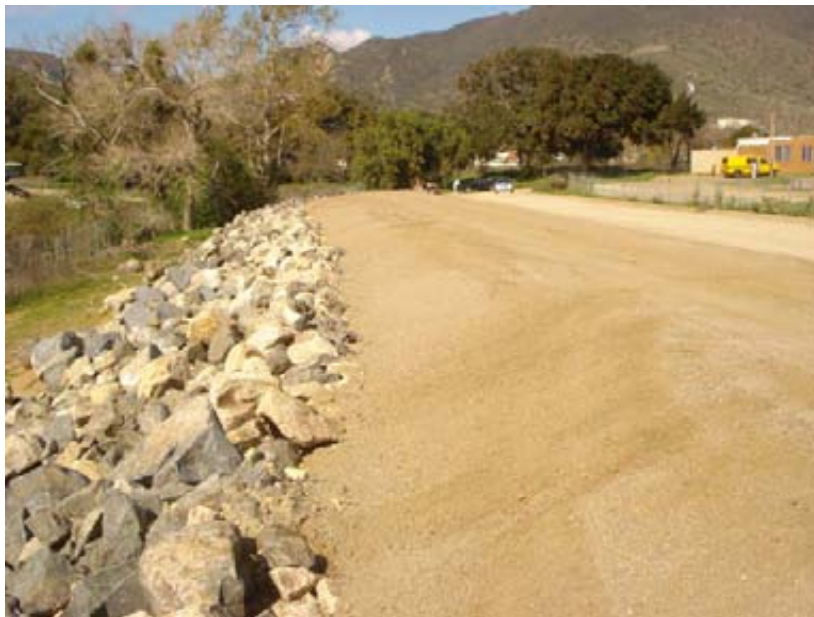
Figure 6 View of Pala Creek and embankment at terminal end of gravity sewer. (2/26/09)
