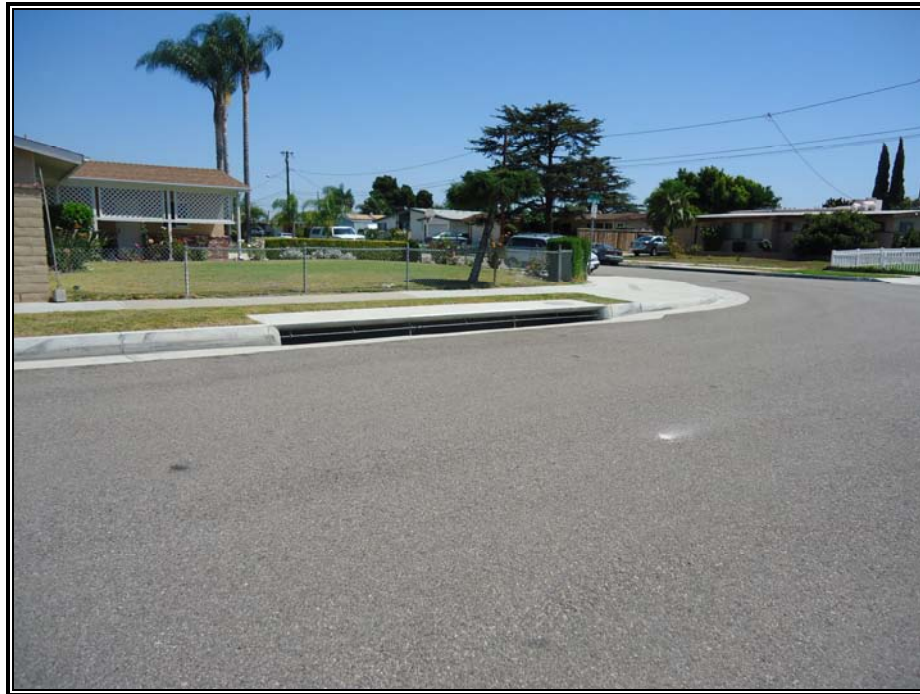
Figure 11 View southeast from Richardson Way and 19 th Street toward existing storm drain inlet.
