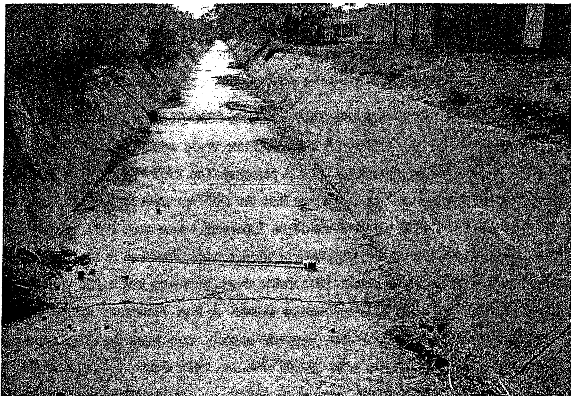
11 12 13 Figure 3.6-3. Concrete Lined Channel along Highway 90 in Sierra Vista]
