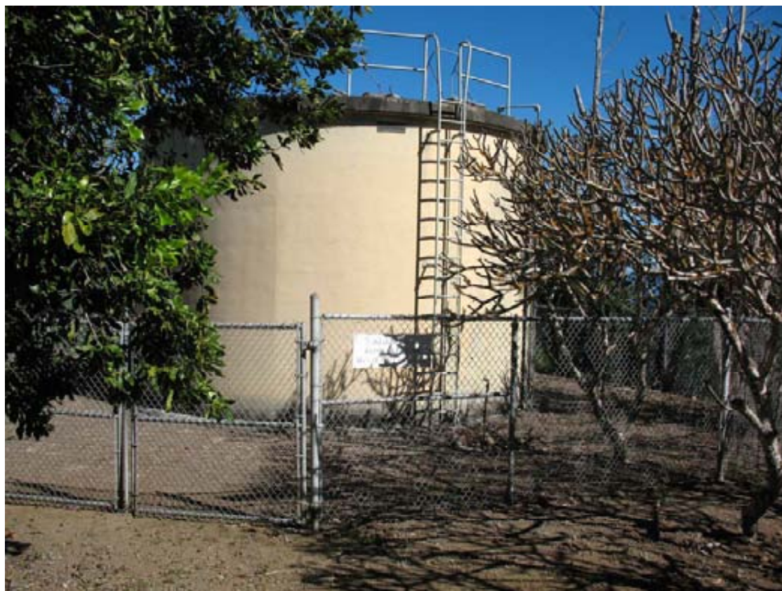
Figure 5. View to north of the existing 50,000 gallon water tank on TMK: 3-4-702:29.
