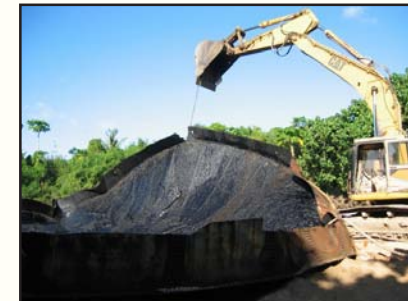
Response teams remove hazardous storage tank
