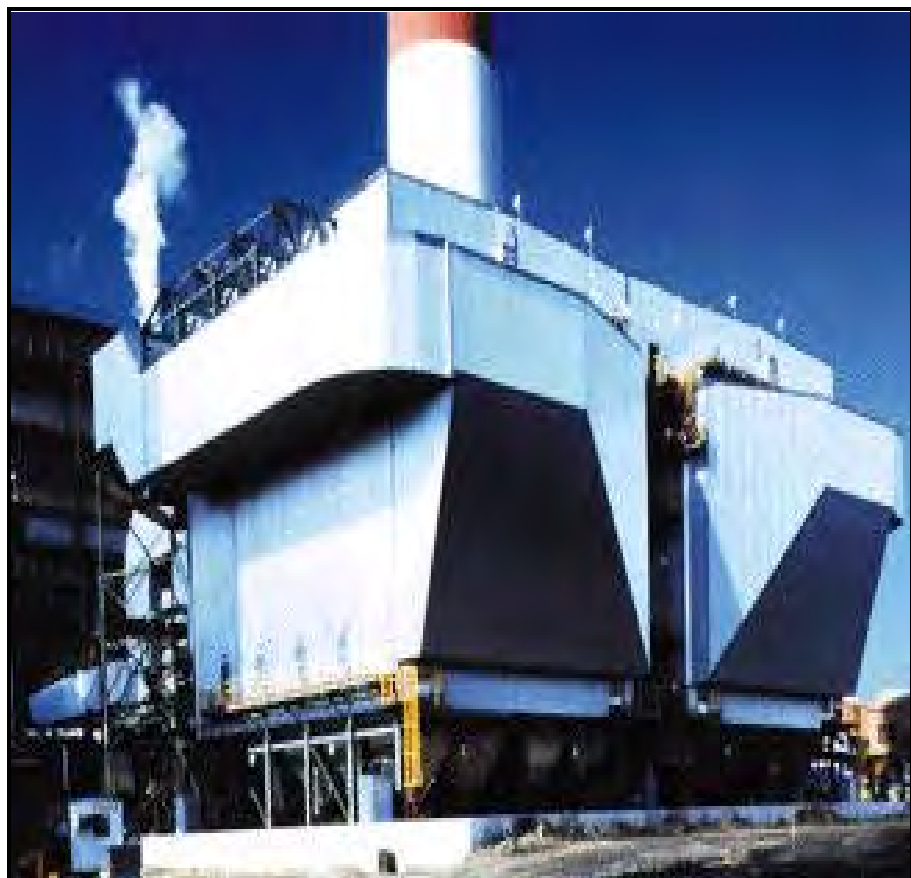
Large ESP at an Electric Utility Facility
