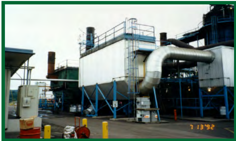
A Pulse Jet Baghouse
