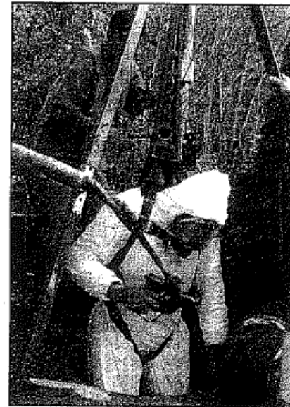
Wayne Allen Daily Times A $90,000 project which began last week in the North Moreland area of Portsmouth will save taxpayers money and meet a request by the EPA at the same time. Manholes in that area are being repaired and will be returned to a "like new" condition. Pictured are Anthony Dye being lowered into the sewer, while Rob Webb lowers him down.
