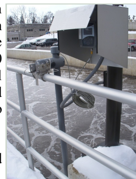
Aeration is energy-intensive process. Close monitoring of dissolved oxygen is essential.
