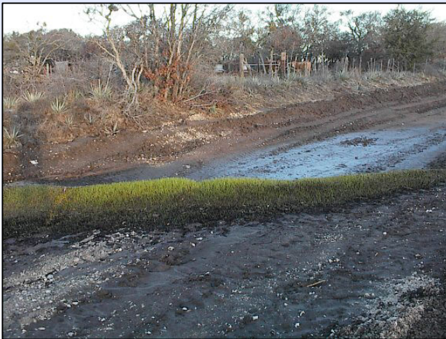
Compost filter berm, US HWY 281 (Texas) on 1/30/2001
