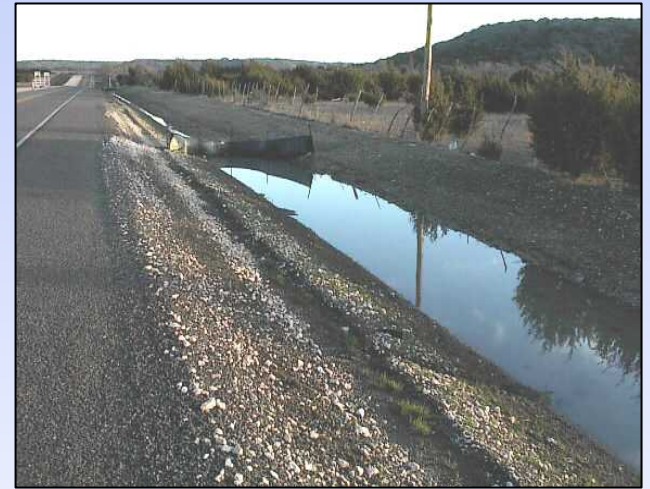
Silt fence, US HWY 281 (Texas) on 1/30/2001
