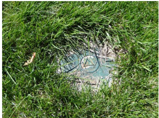
A flush mounted monitoring well located in Bayfront Park
