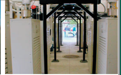
Microturbines in the methane co-generation plant.
