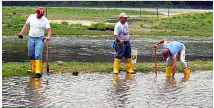
Ecosystem restoration activities, such as planting aquatic vegetation, have transformed areas excavated during remediation into functional habitats. (Source: U.S. DOE)
