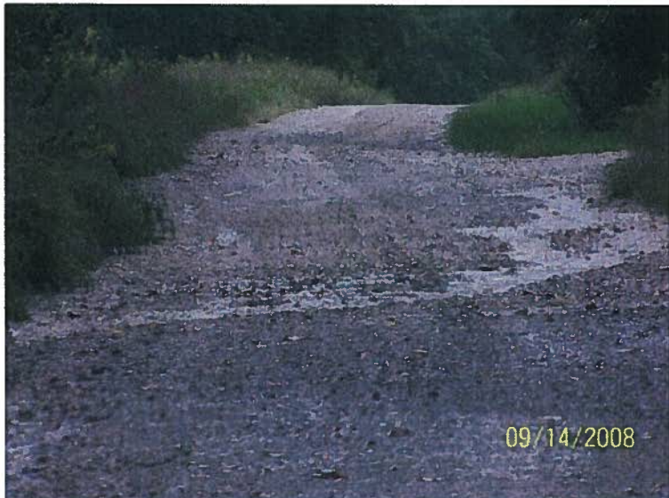
WATER RUNNING OUT OF THE HILLTOP CONFINEMENT DRIVEWAY NEXT TO CULVERT RUNNING DOWN THE ROAD TO SUGARCREEK IN ABOVE PICTURE
