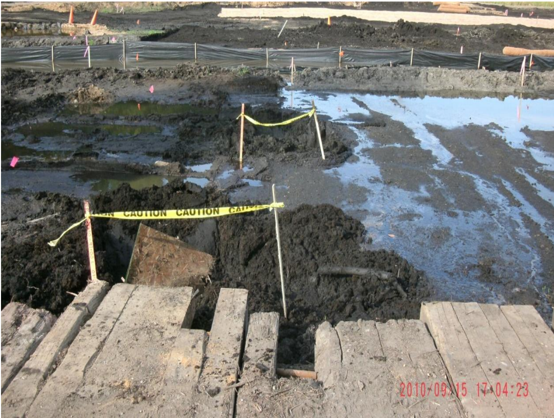
47+00L – 47+50L: Looking toward Talmadge Creek at 6-hour test and 48-hour observation pits (September 15, 2010)
