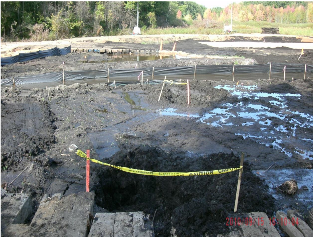
47+50L – 48+00L: Looking toward Talmadge Creek at 6-hour test and 48-hour observation pits (September 15, 2010)
